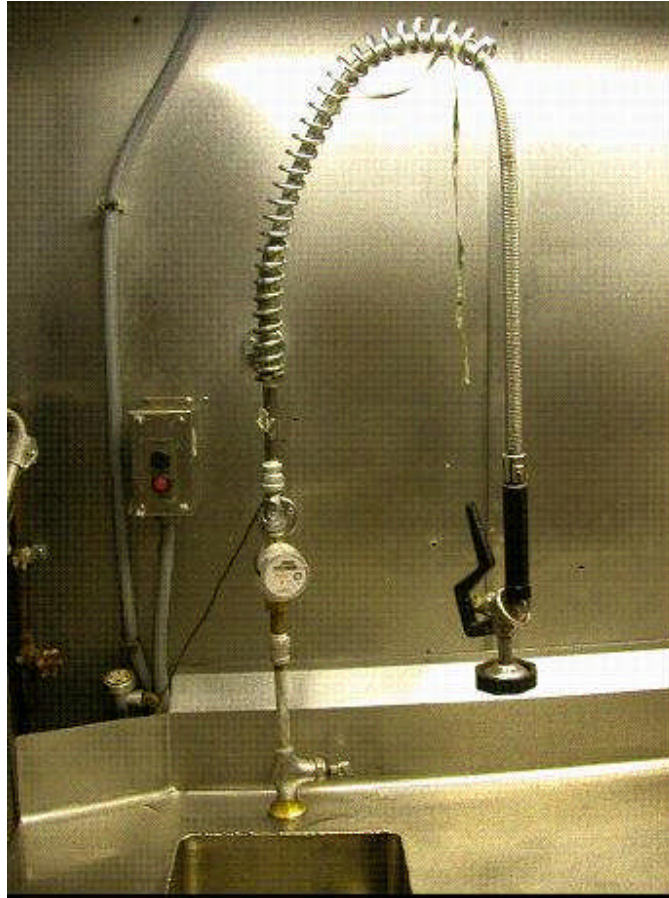
Figure 12. Pulse-Generating Meter Installed on Riser to PRSV
