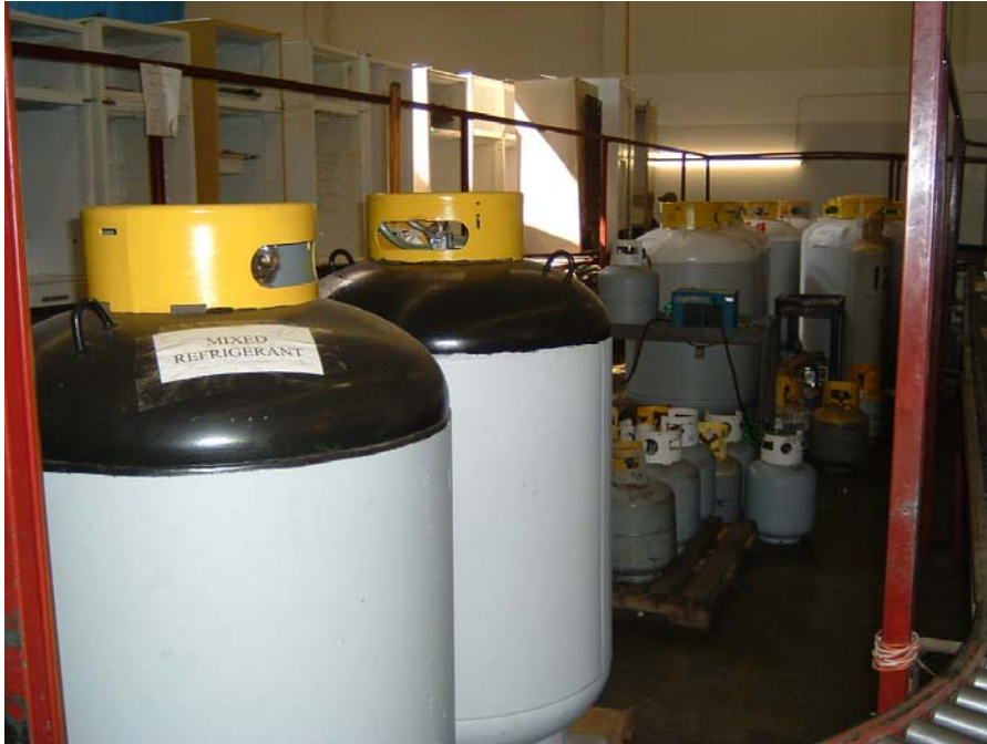
Figure B-8 Recovered CFCs Are Stored in Large Containers
