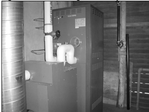
Figure 3.9 Site #115 High Efficiency Boiler
