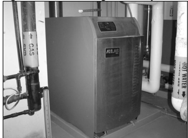
Figure 3.10 Site #215 High Efficiency Boiler
