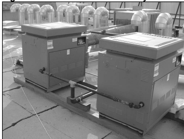
Figure 3.6 Site #164 Low Efficiency Boiler
