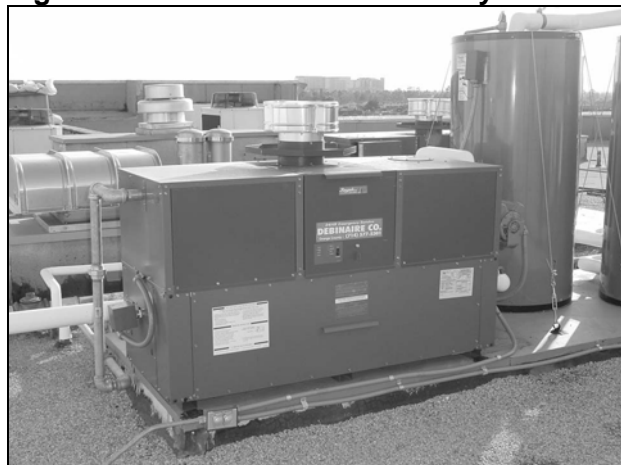
Figure 3.5 Site #157 Low Efficiency Boiler
