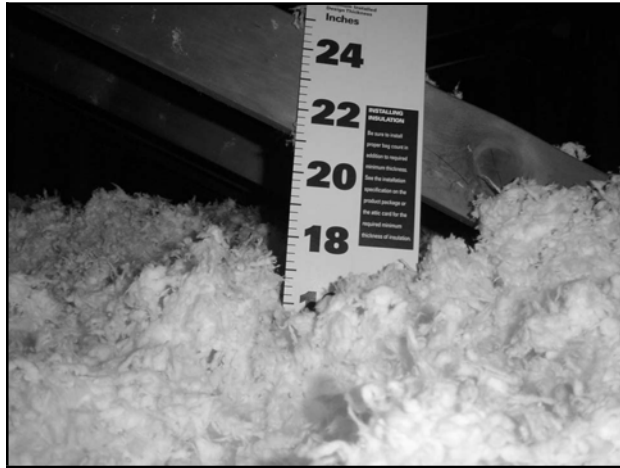
Fig. 3.7 Midway-Capri R30 Attic Insulation
