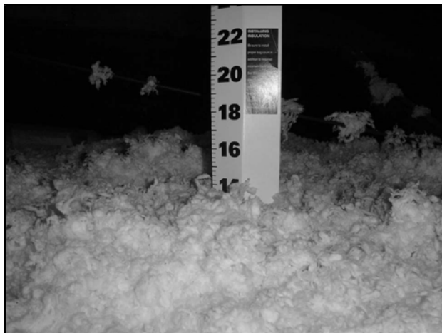
Fig. 3.9 Orange Tree R30 Attic Insulation
