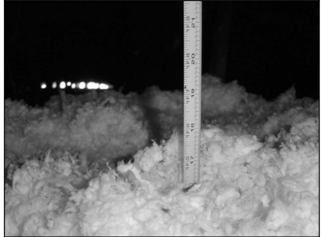
Fig. 3.2 Flanders R30 Attic Insulation
