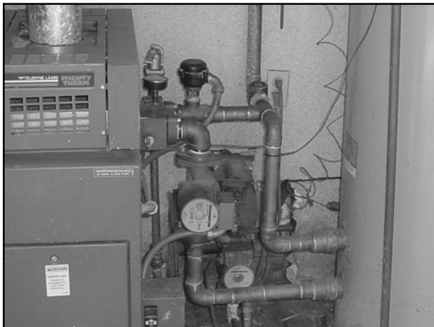
Fig. 3.5 Flanders No Pipe Insulation
