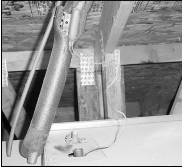
Figure 2.3 Uninsulated TXV Bulb in Attic
