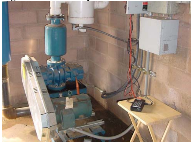
Figure 6.3 New Pump w/VFD at Site #1
