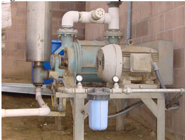
Figure 6.2 Old Vacuum Pump at Site #1
