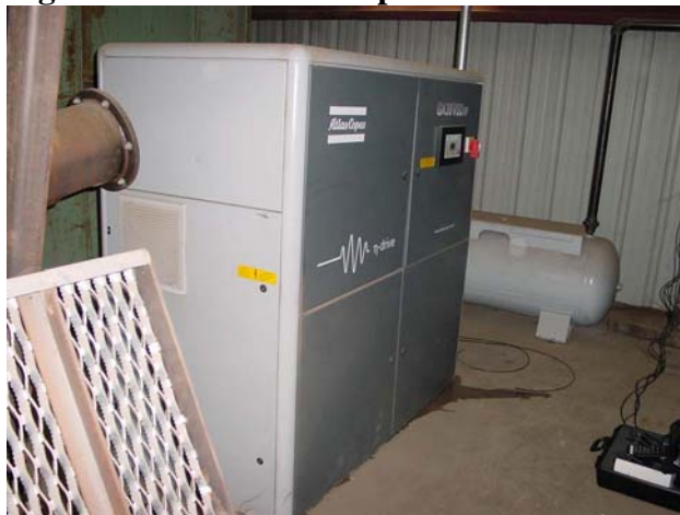
Figure 6.7 VSD Air Compressor at Site #6
