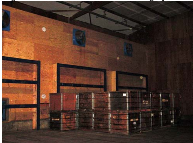
Figure 5.3 New Internal Air-Cooling System
