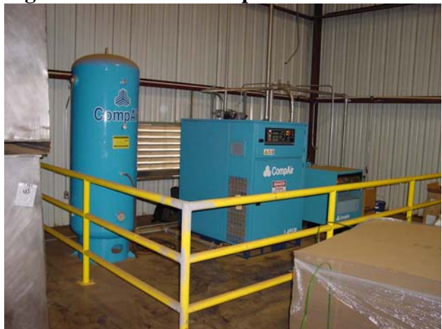
Figure 6.6 VSD Air Compressor at Site #4
