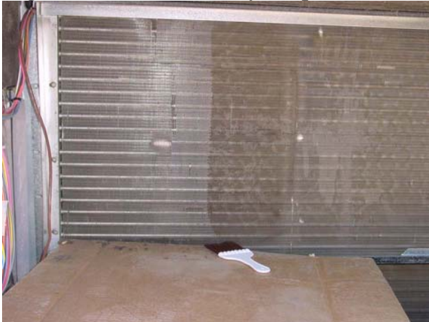
Figure 4.7 Clean and Dirty Evaporator Coil
