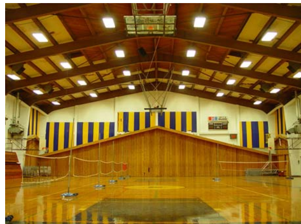
Figure 2. Post-Retrofit T5 6-Lamp Fixtures
