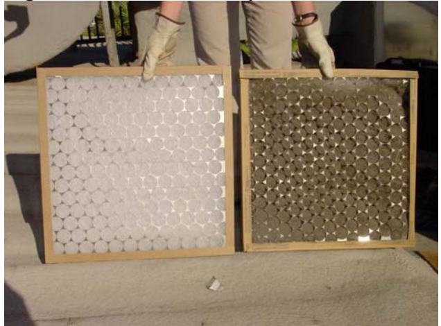
Figure 2.8 Clean and Dirty Air Filter
