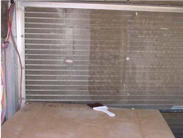
Figure 2.7 Clean and Dirty Evaporator Coil
