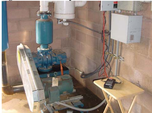
Figure 2.3 New Pump w/VFD at Site #1
