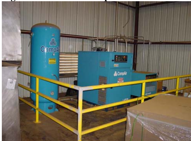
Figure 2.6 VSD Air Compressor at Site #4
