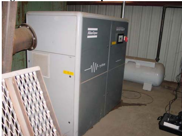
Figure 2.7 VSD Air Compressor at Site #6
