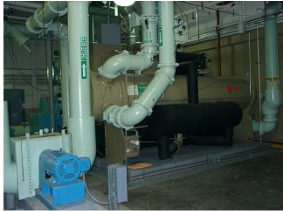
New Chiller (Right Side)
