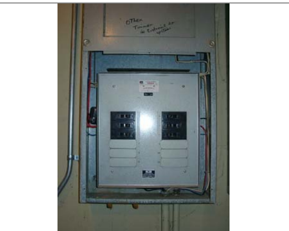
Garage Power Room Panel LA
