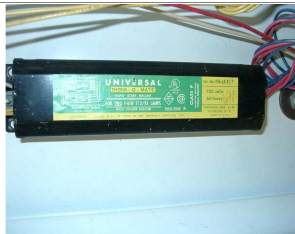
Boiler Room 4-lamp Fixture Ballast
