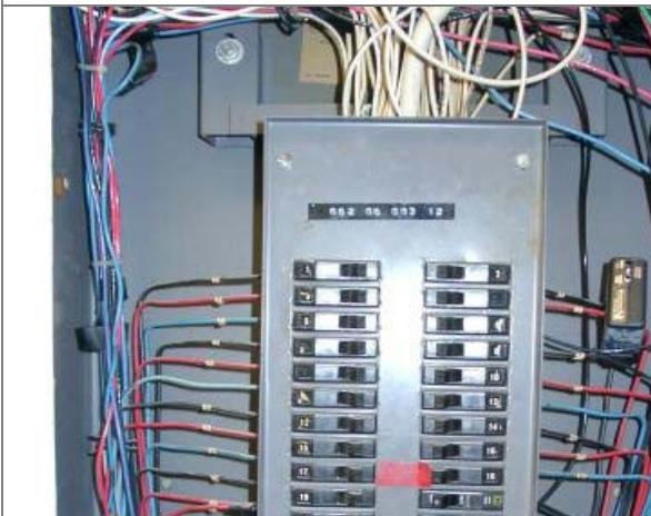
Panel C Breaker Panel
