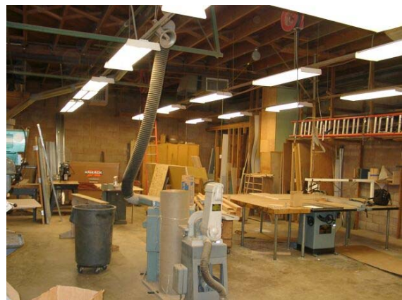
Carpenter Shop Light Fixtures
