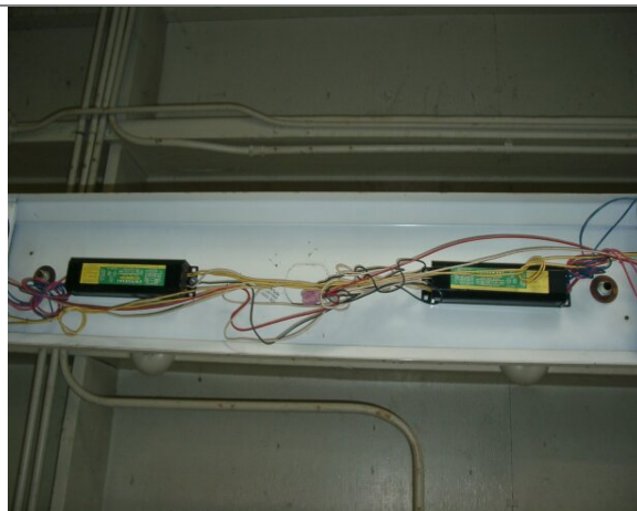
Boiler Room 4-lamp Fixture
