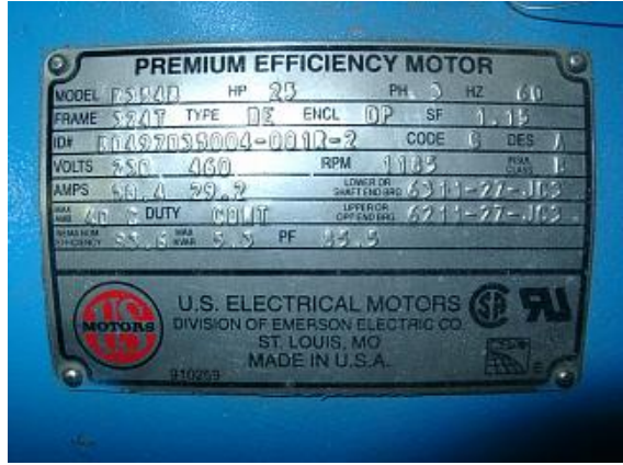
New Chiller 25hp Motor Nameplate
