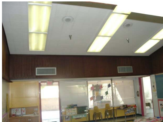
Classroom #2 Ceiling Fixtures
