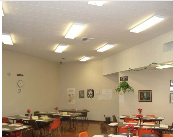
Dining Room T-8 Lighting Fixtures
