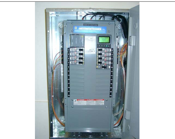
New Lighting Breaker Panel E
