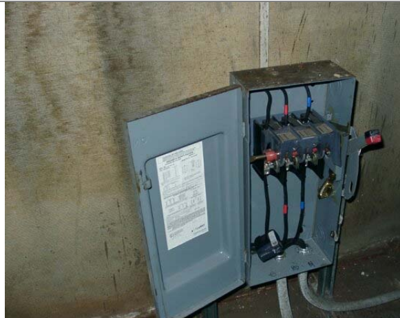
Room C-25 Right Side AHU Disconnect
