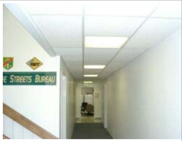
Hallway 2x2 Fluorescent Fixtures
