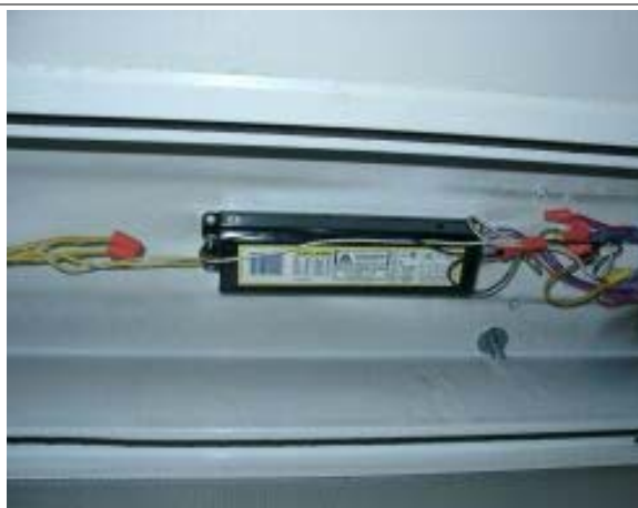
Rest Room 1x4 Fixture Ballast
