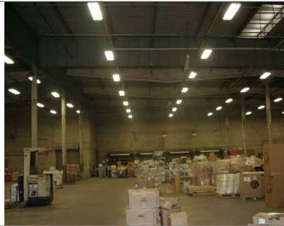
T-5 4-Lamp Fixtures (Warehouse)
