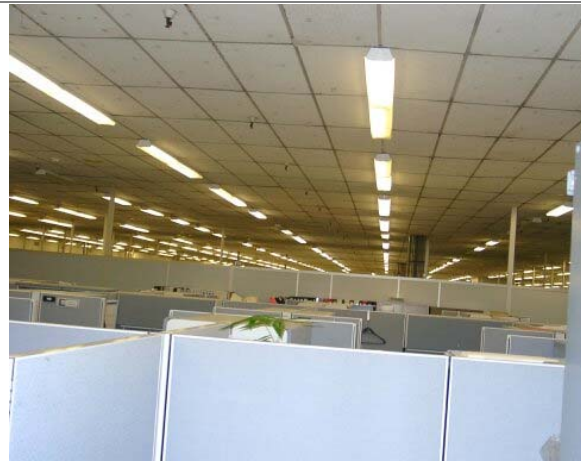
2 nd Floor Open Area Light Fixtures
