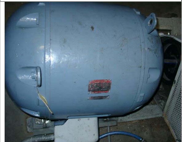
W-93 Room 4 AHU Motor
