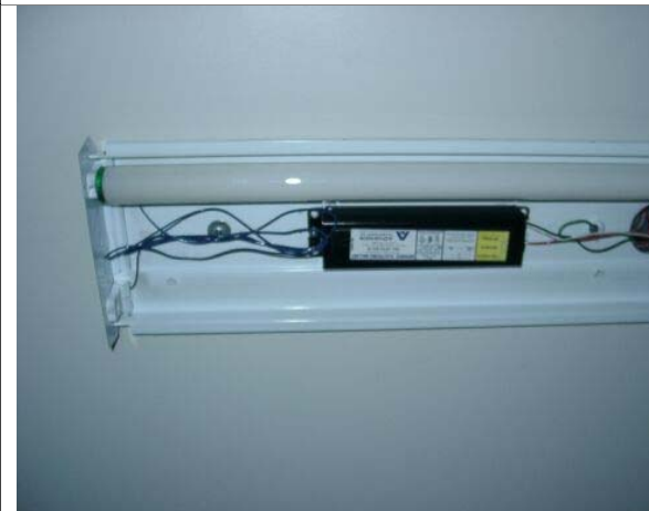
2-Lamp Light Fixture And Ballast
