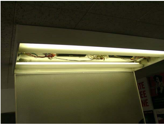
Lobby, 4-lamp Fixture (Near Reception)
