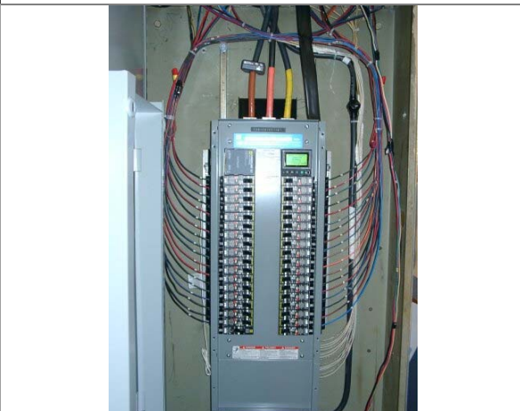
New Lighting Breaker Panel 2J235 Upstairs
