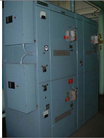
4160 V Panel for Chillers
