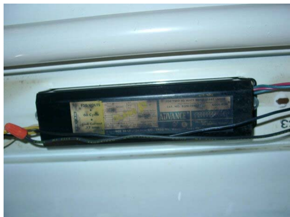
Boiler Area Wrap Fixture Ballast
