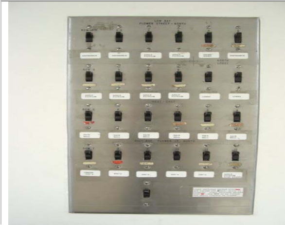
Library Light Switches (Right Side)
