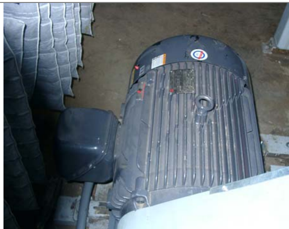
Room C-25 Right Side New Motor
