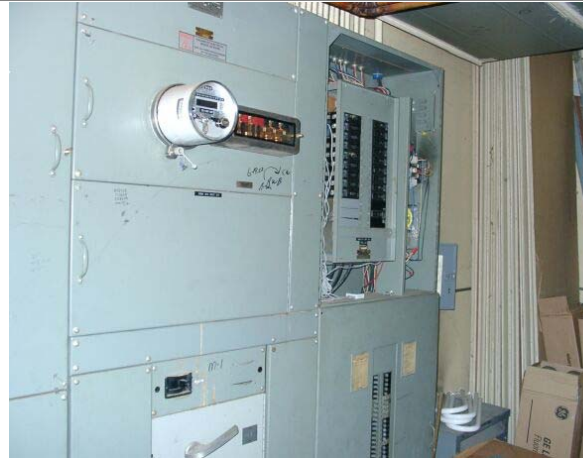
Equipment Room Electrical Panels
