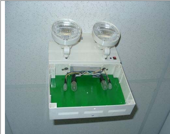
Exit Sign – Gain Claims Office
