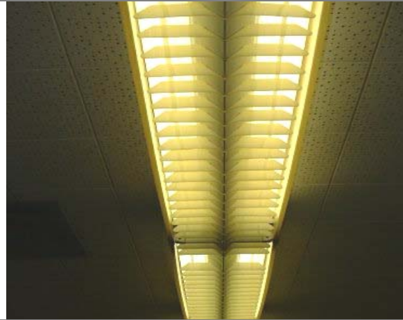
Old T12 Fixtures in Gun Training Classroom
