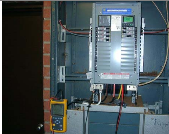
New Panel MH
