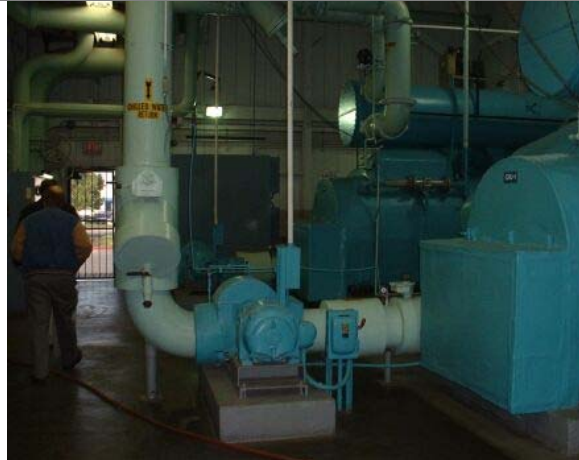
CRU-1 and CRU-2 Chiller Room View
