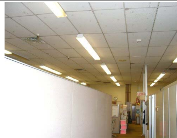
Downstairs Open Area Fixtures Near Panel F
