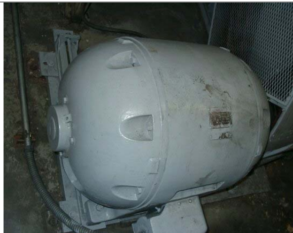
W-81 Room 3 AHU Motor
