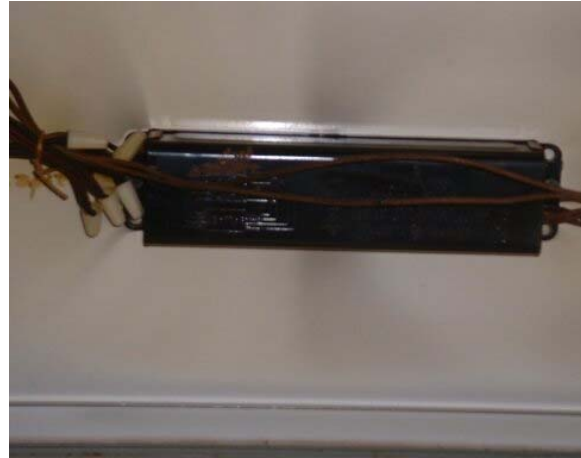
Damaged Old T12 Ballast
