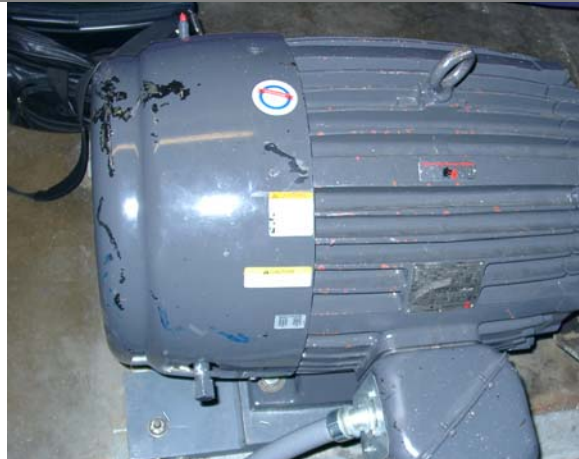
W-93 Room 4 AHU Motor (New)
