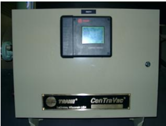
New Chiller Control Panel
