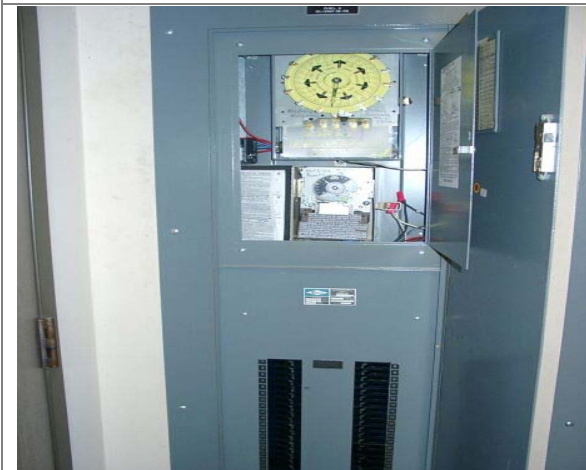
Contactor that feeds top half of panel A
