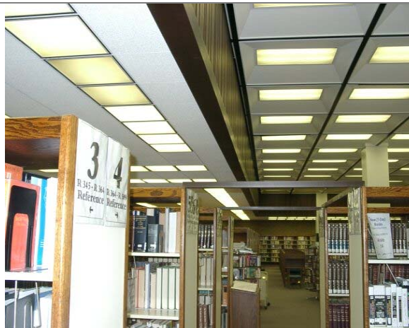
Main Library 2-lamp and 4-lamp 4-Foot Fixtures
