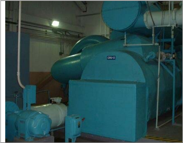
Trane CRU-2 Chiller
