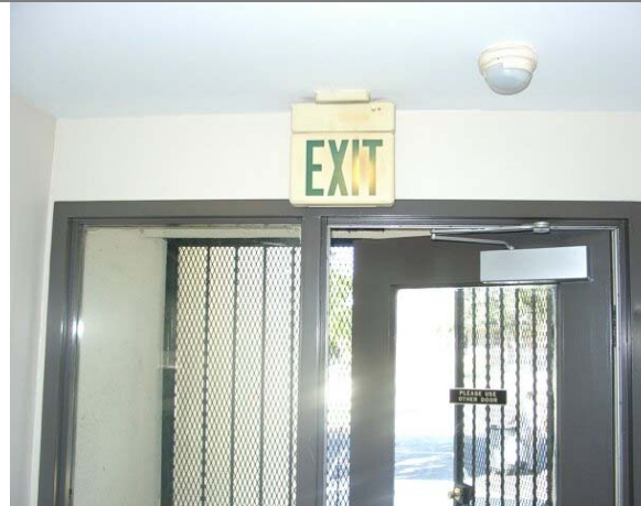
Powered Exit Sign Location
