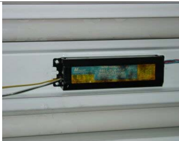
Another F40T-12 Ballast
