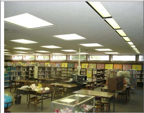
Children's Library, 4 x 4, 8-lamp Fixtures
