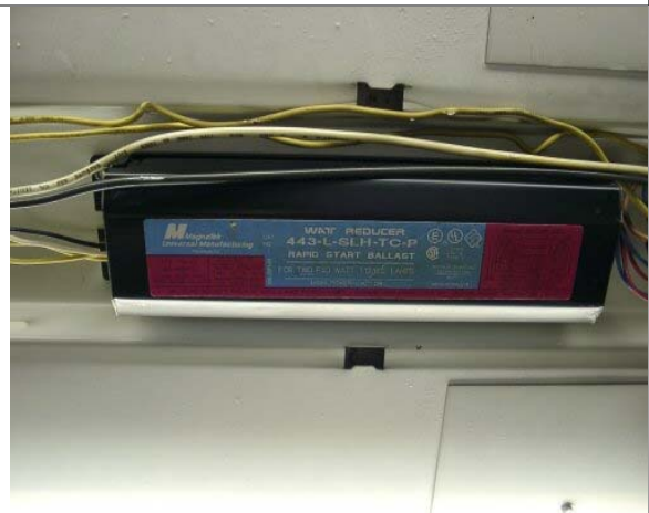
4 Lamp Fixture Ballast
