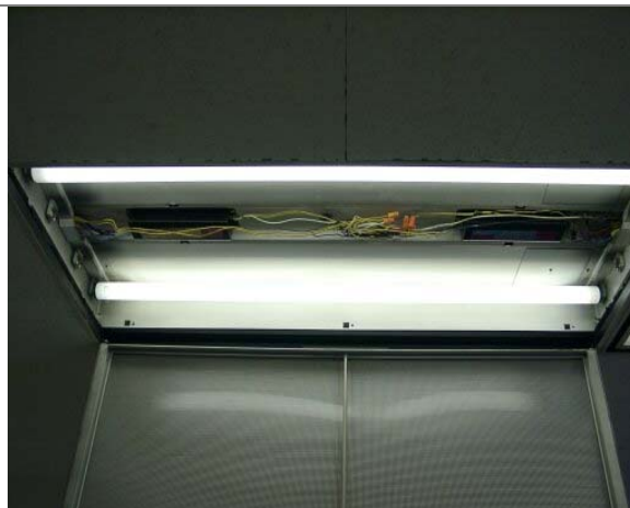
4 Lamp Fixture and Ballasts
