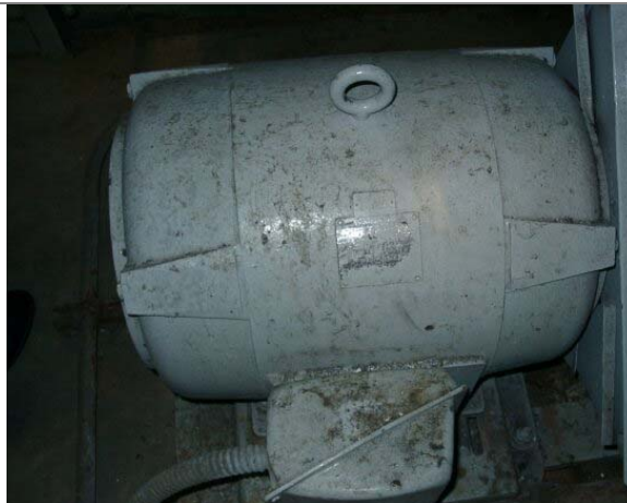
Upstairs SE Corner AHU Motor
