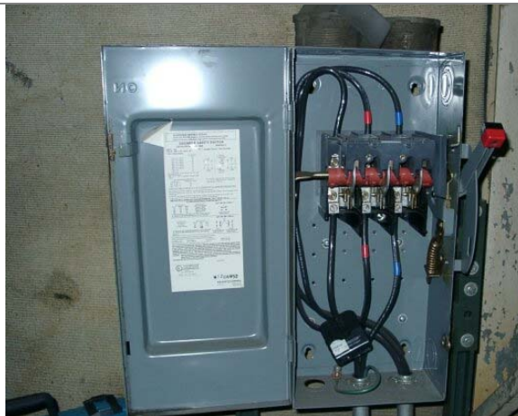
W-81 Room 3 AHU Disconnect
