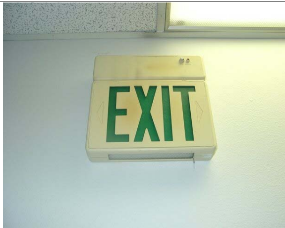
Powered Exit Sign (1 Of 3)
