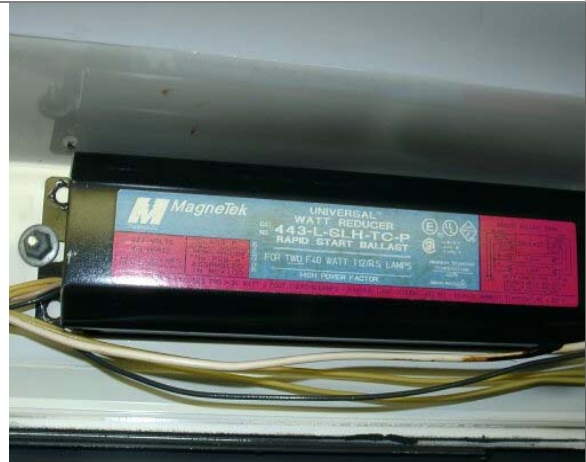
Main Library 4x4 Ballast
