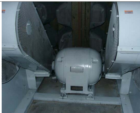
Room 044 AHU Dual Shaft Motor
