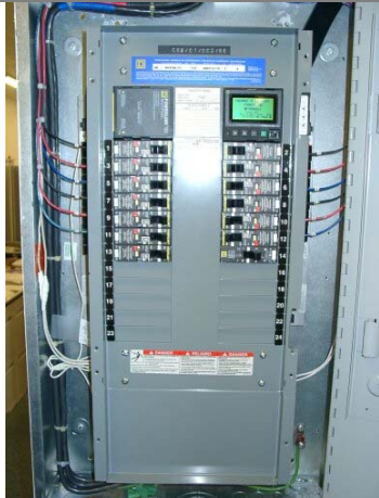
New Lighting Breaker Panel G-69
