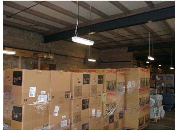
Warehouse 2-foot Fluorescent Light Fixtures
