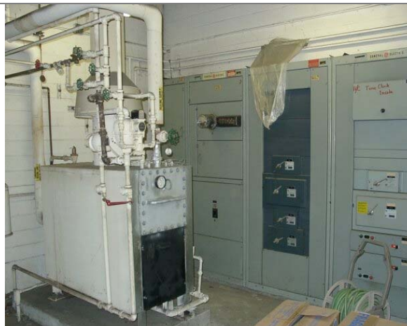
The Equipment Room Boiler And Main Electrical Panels
