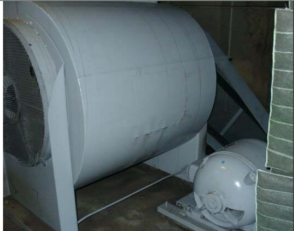
Room C-25 Left Side AHU
