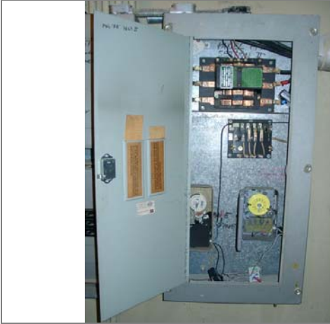
Garage Power Room Panel PA Section 2 With Datalogger
