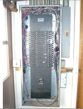
Warehouse Main Breaker Panel A
