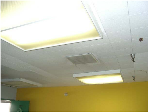
Small Classroom Surface Mounted 4-lamp Fixtures
