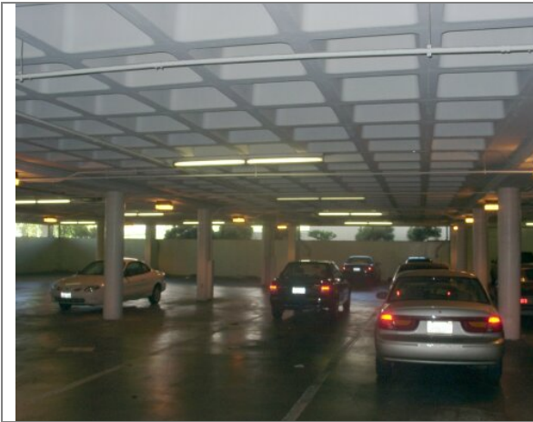
Parking Garage Lighting
