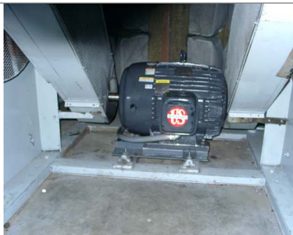
Room 044 AHU New Motor
