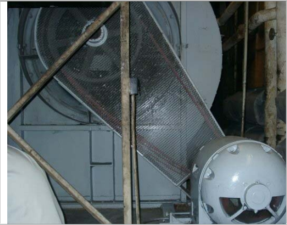
W-81 Room 3 AHU
