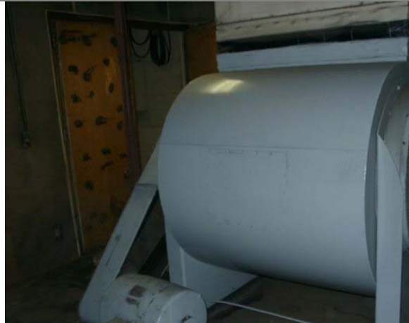
Room C-25 Right Side AHU
