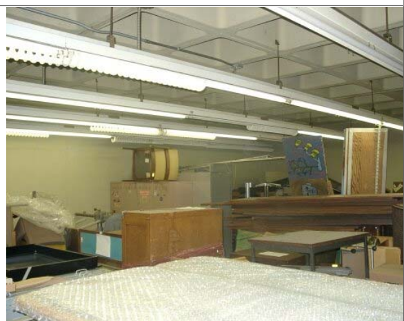
Garage Level Storage Room Light Fixtures
