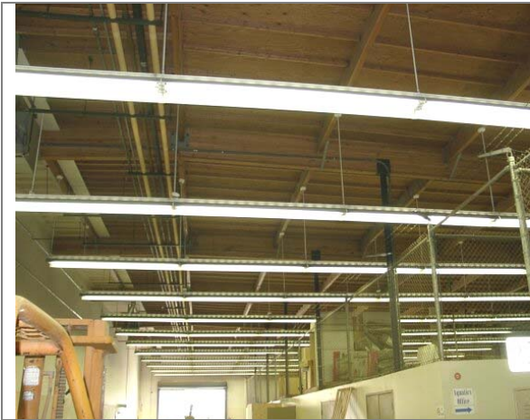
Main Warehouse Old T12HO Fixtures
