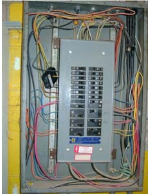
Carpenter Shop Breaker Panel with Datalogger
