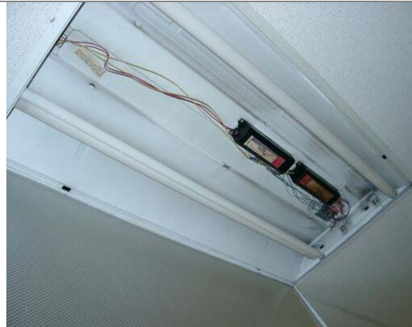
Fixture – 2x4 Ballast Locations
