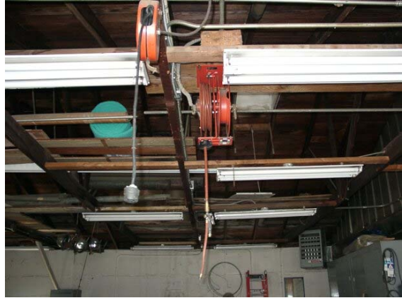
Carpenter Shop Fixtures
