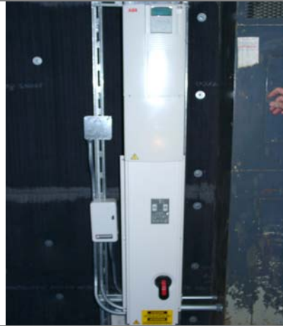
Auditor Room New VFD System
