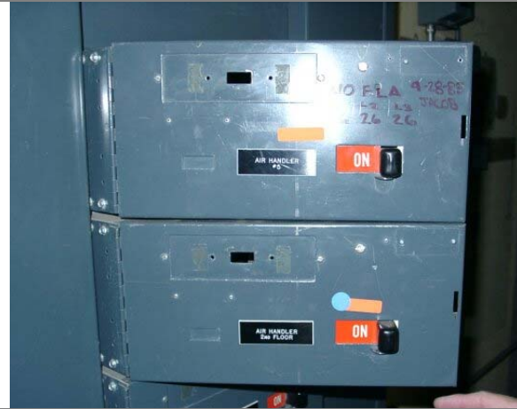
Room C-54, AH-3 and AH-5 Disconnects
