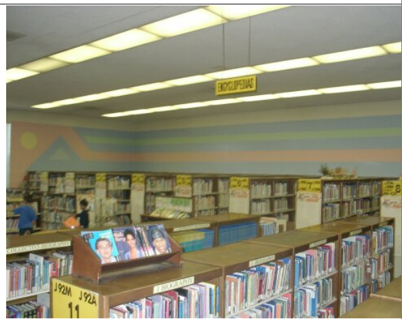
Children's Library Light Fixtures
