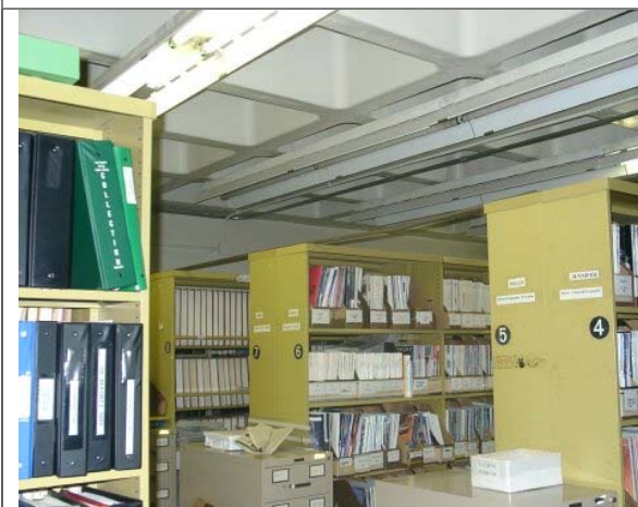
Downstairs Book Storage Light Fixtures
