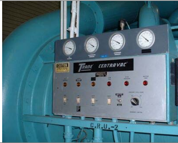
Trane CRU-2 Controls
