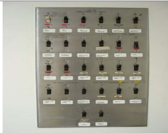
Library Light Switches (Left Side)
