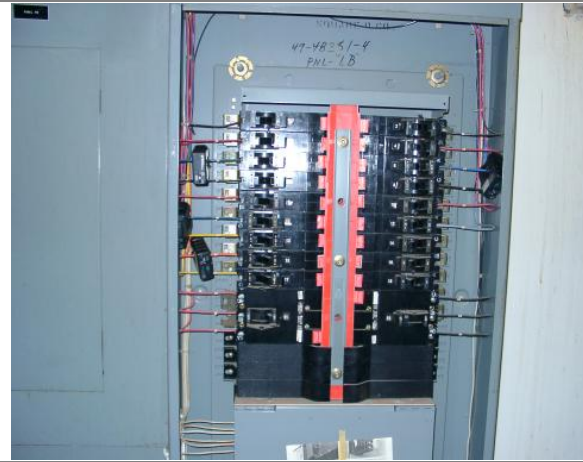
Panel LB in Main Vault with Dataloggers Installed
