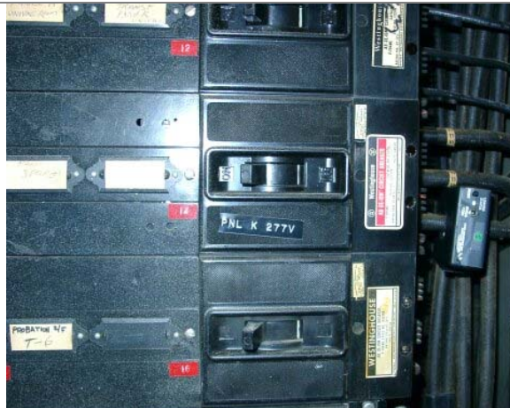
Datalogger On Breaker For Panel L
