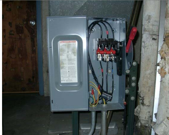
Room 044 AHU Disconnect
