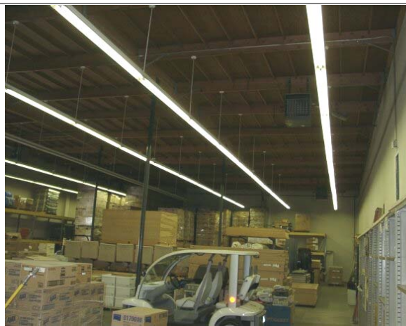
Shipping Warehouse Old T12HO Fixtures
