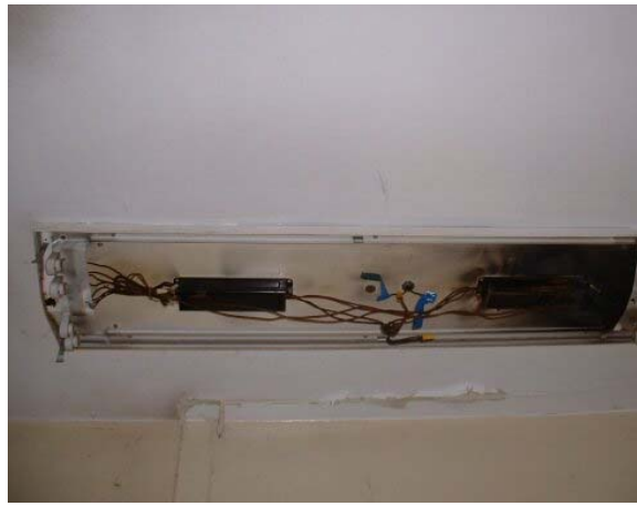
Damaged Old T12 4-Lamp Fixture
