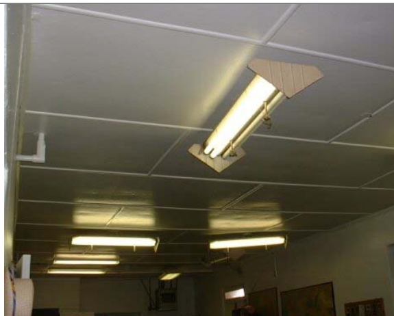
T12 Fixtures for Office Next to Car Wash
