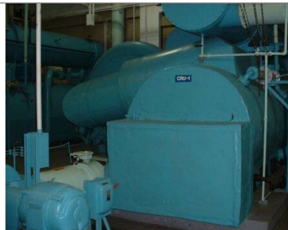
Trane CRU-1 Chiller
