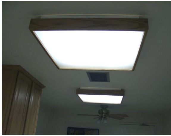
Kitchen U-Bend Fixtures
