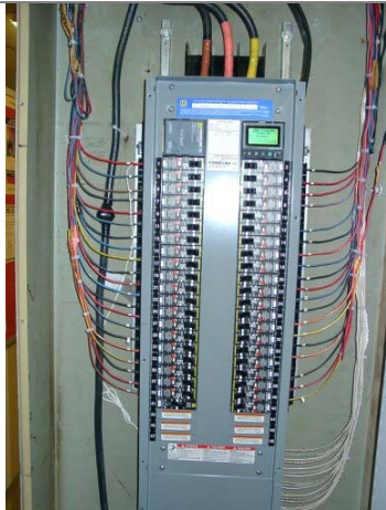
New Lighting Breaker Panel F
