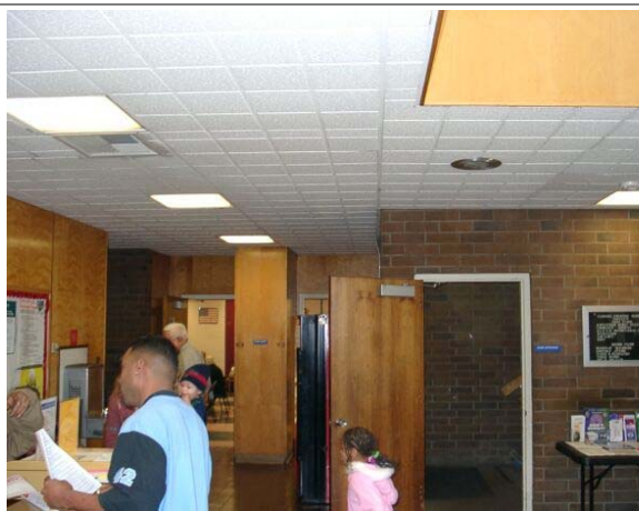
Lobby Light Fixtures
