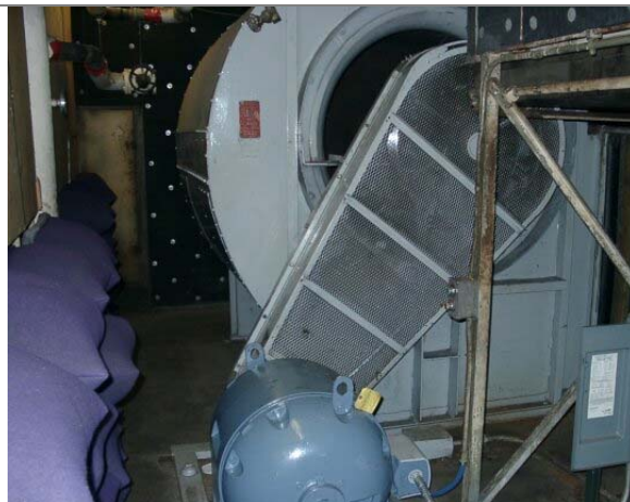
W-93 Room 4 AHU
