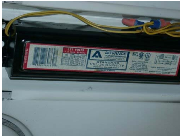
2 Lamp U-Bent Fixture Ballast
