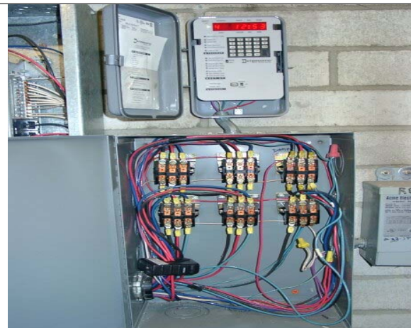
Lighting Relay Panel with Data Logger
