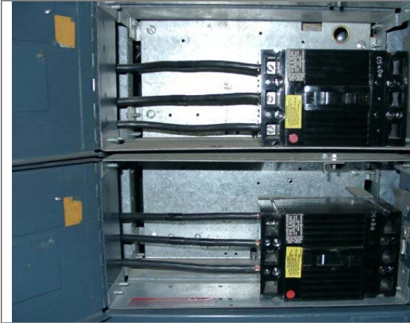
Room C-54, AH-3 and AH-5 Breakers
