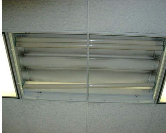
Another Picture of a 4-lamp 4-Foot Fluorescent Fixture
