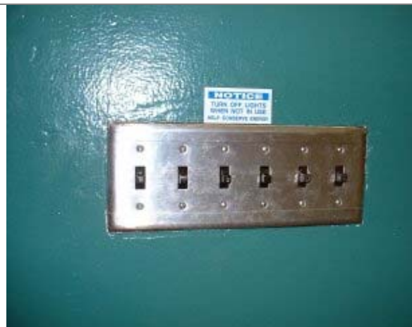
Gym Lighting Switches
