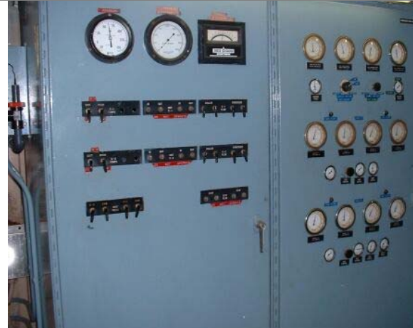
Control Panel in CRU-1 and CRU-2 Room
