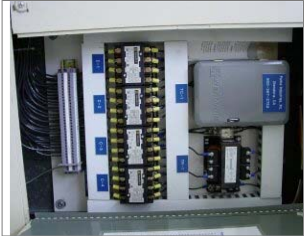
Parking Lighting Control System
