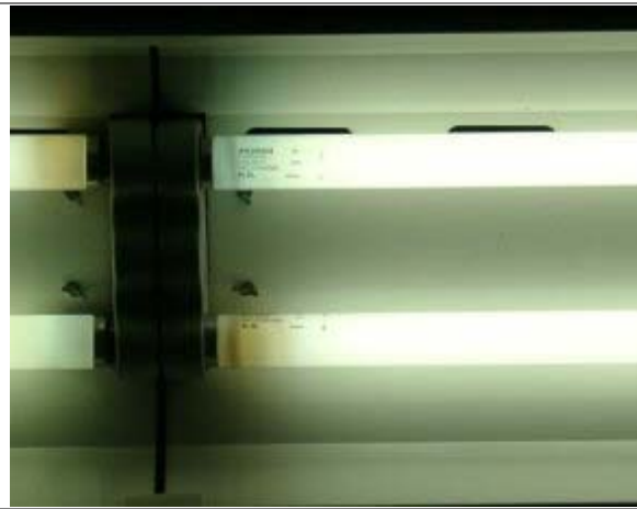
Close Up Photo Of 2-lamp Old T12HO Fixtures
