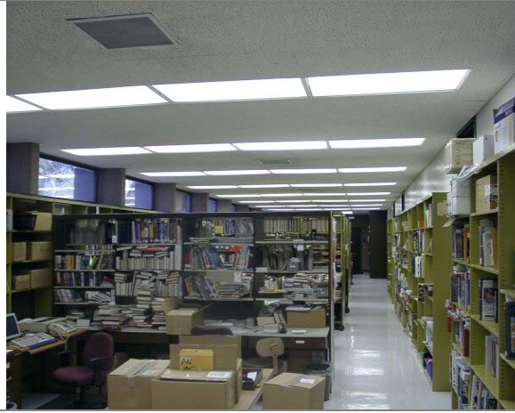
2 x 4 Troffers In The Work Room
