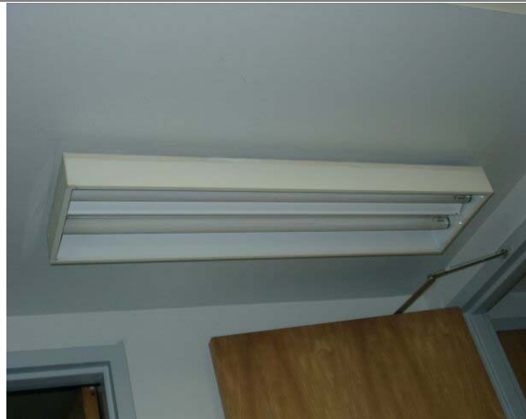
Office Hallway 2-lamp Fluorescent Fixture
