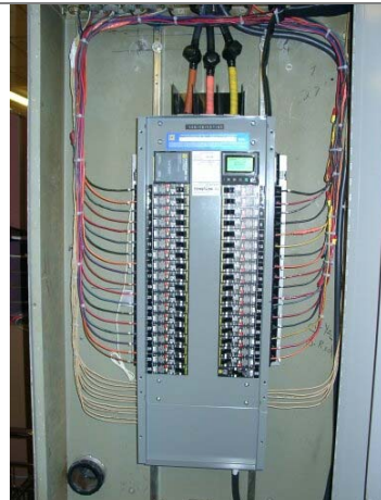
New Lighting Breaker Panel 2E235
