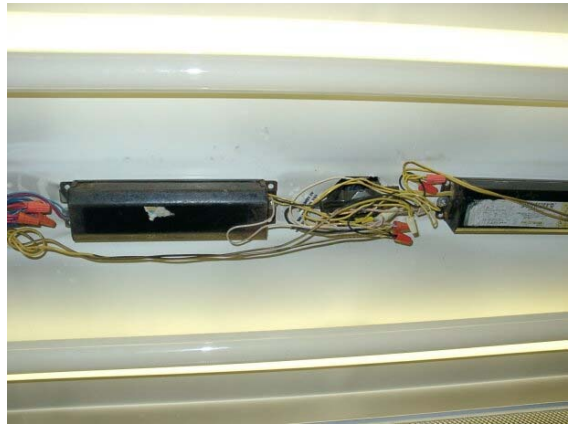
Lobby Fixture Ballasts (Near Reception)
