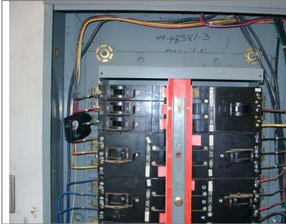
Panel LA in Main Vault with Datalogger Installed
