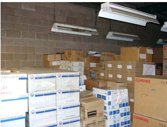
Warehouse Light Switch Located Behind Pallets On Wall That Cannot Be Operated
