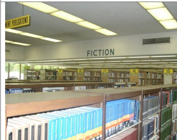
Main Library Light Fixtures
