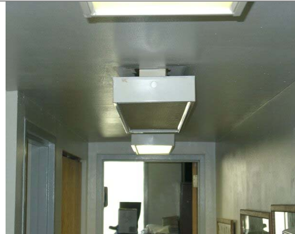
Office Surface Mount 2-lamp Fixtures
