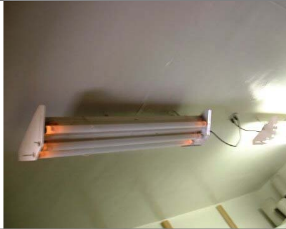
Old T12 Fixture Failing to Light Properly
