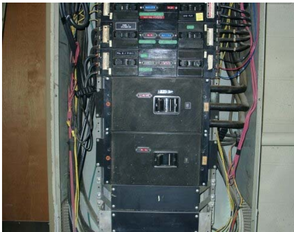
4160 Vault PP4 Panel With Dataloggers
