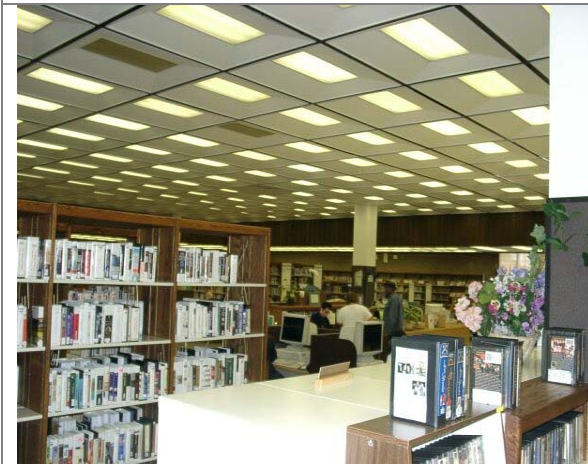
Main Library 2-lamp 4-Foot Fixtures
