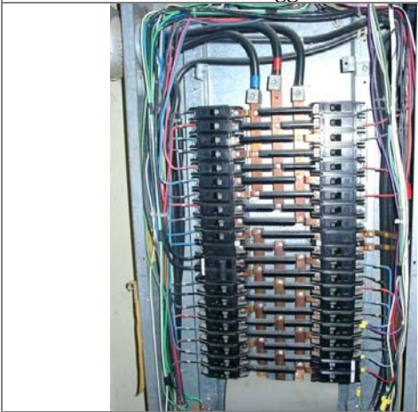
Garage Power Room Panel PA Split Bus
