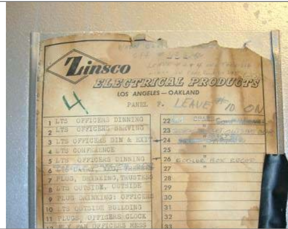
Kitchen Area Breaker Panel F Legend
