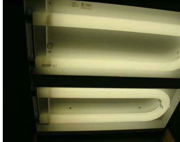
Kitchen U-Bend Fixtures
