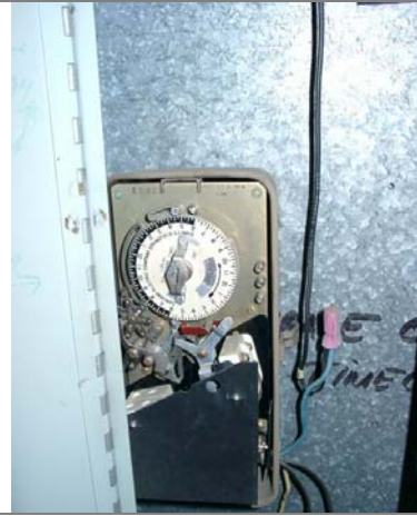
Garage Power Room Timer for T8 Lights
