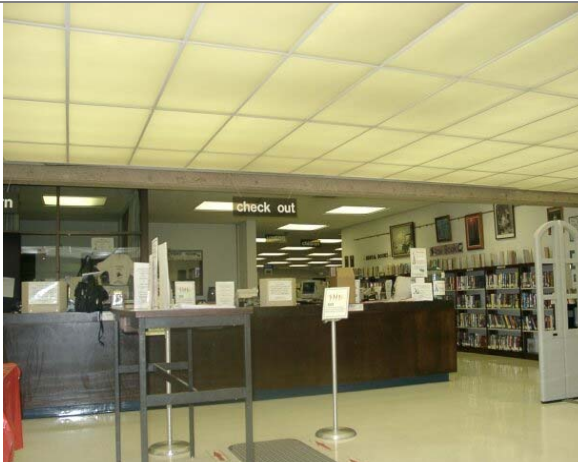
Lobby Lighting, 1 x 4 Mixed Ballast Fixtures
