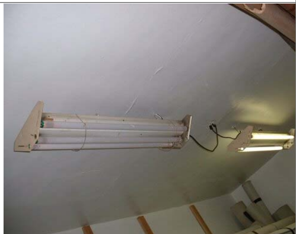
More T12 Fixtures in Office Next to Car Wash
