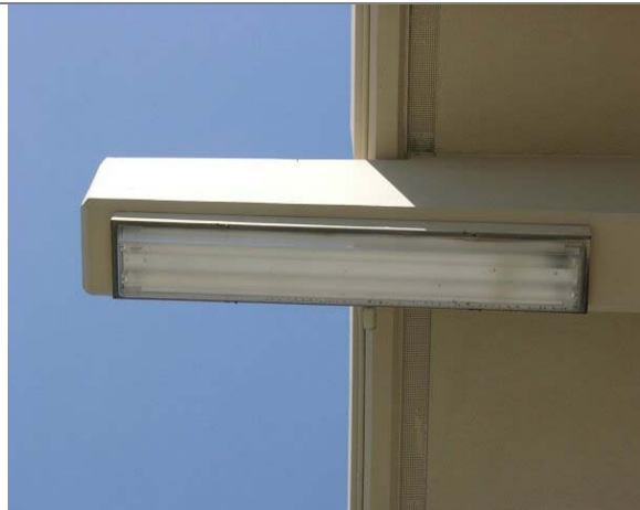
Outdoor 4-foot 2-lamp Fixture (On Beams)
