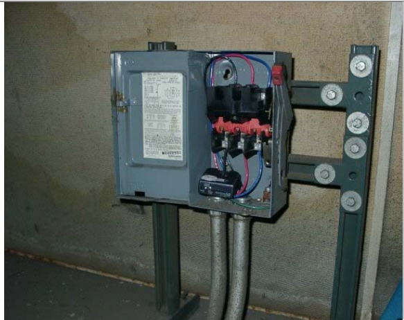
Room C-25 Left Side AHU Disconnect
