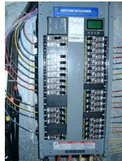
New Lighting Breaker Panel L-1
