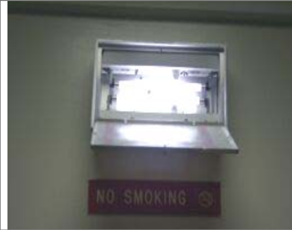
Fluorescent Exit Sign
