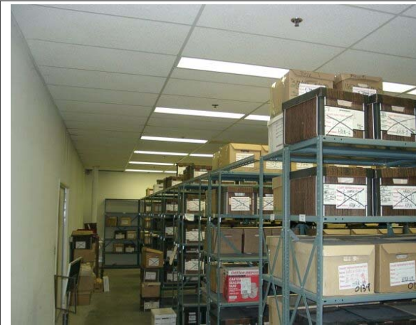
More Storage Room Lighting Fixtures
