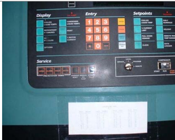
York 750 Control Panel
