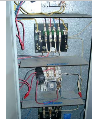
Garage Power Room Contact Timer (middle) With Datalogger
