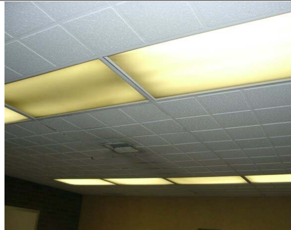
Fixtures in Meeting Hall
