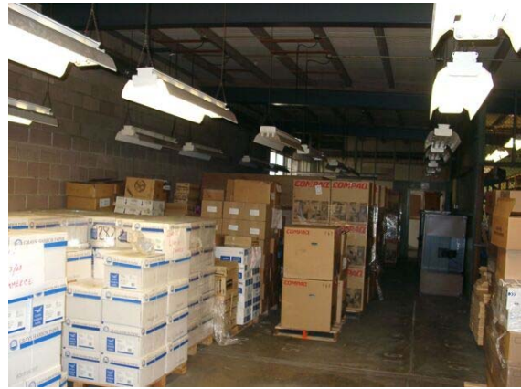
Warehouse Light Fixtures
