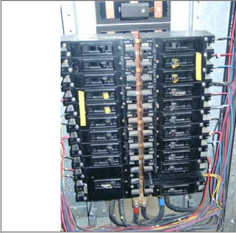
Garage Power Room Panel LE
