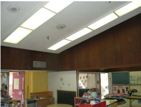
Classroom #1 Ceiling Fixtures
