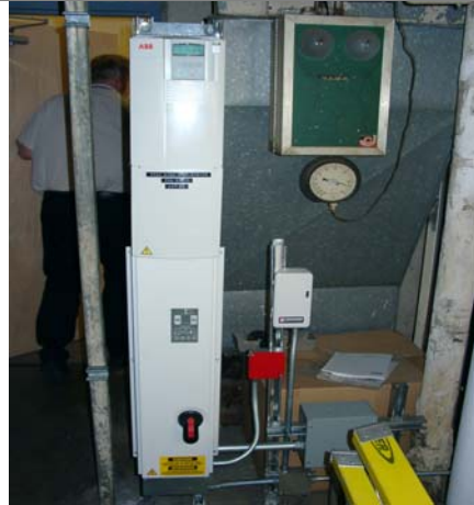
Room 044 AHU New VFD System
