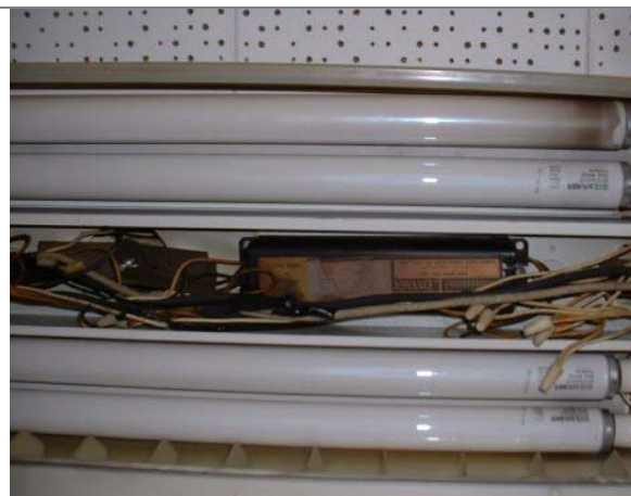
Magnetic Ballast T12 4-Lamp Fixture
