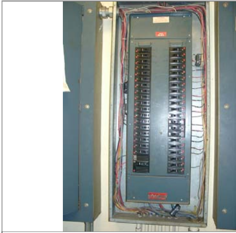
Lighting Panel and Data Loggers
