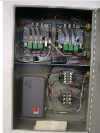
Upstairs Lighting Contactor
