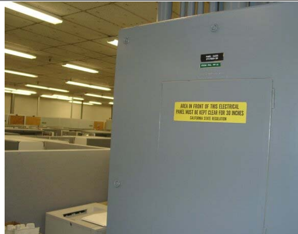
Old Lighting Breaker Panel 2J235 Upstairs
