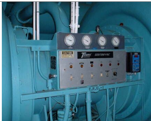
Trane CRU-1 Controls
