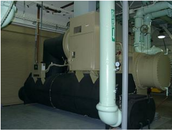
New Chiller (Left Side)
