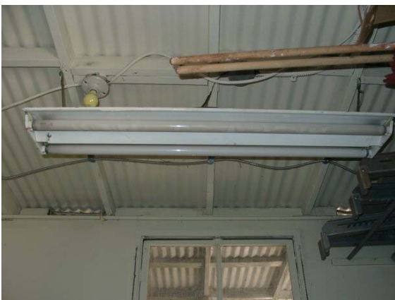
Boiler Area Wrap Fixture
