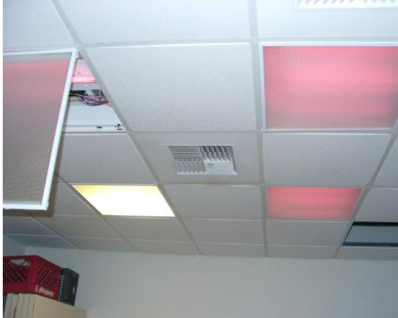
Defective T8 U-Tube Lamps In Machine Shop
