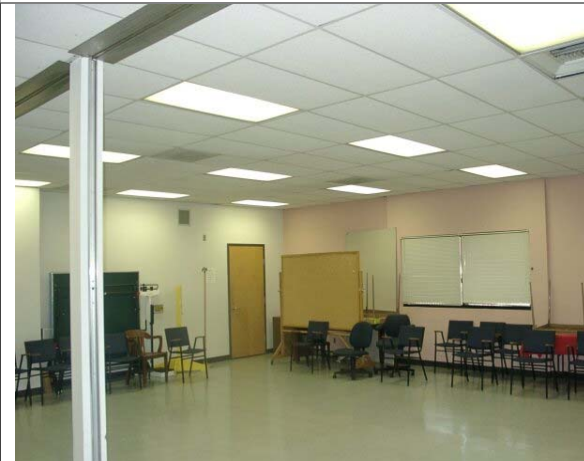
Auditorium T-12 Lighting Fixtures
