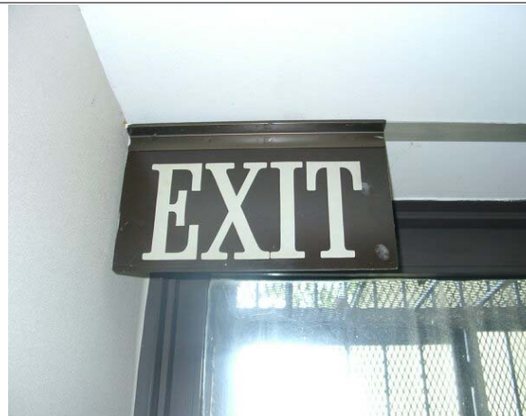
Non-Powered Exit Sign (1 Of 3)
