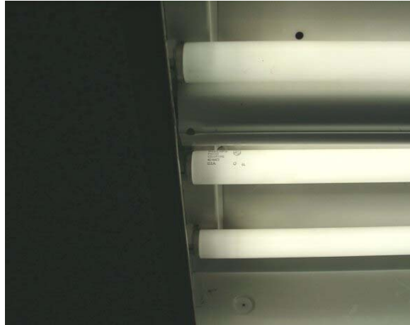
4-lamp Office Light Fixtures (40 Watt Lamps)
