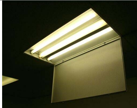
Fixture – 2x4 Fixture Style
