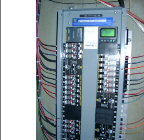
New Lighting Breaker Panel N
