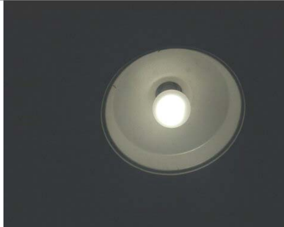
Equipment Room Incandescent Fixture
