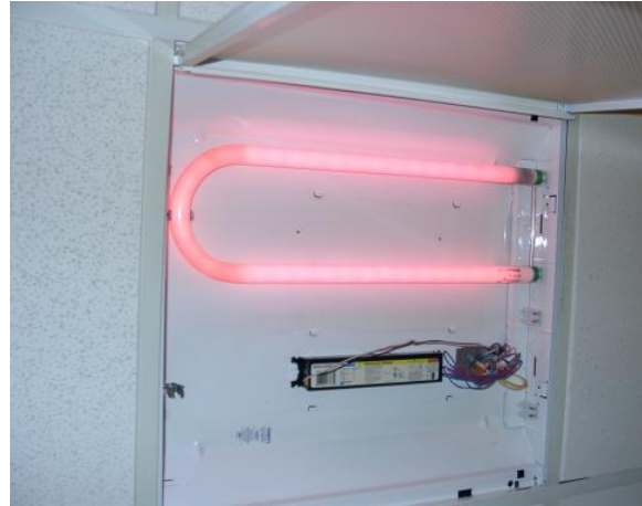
Defective T8 Lamp In U Tube Fixture
