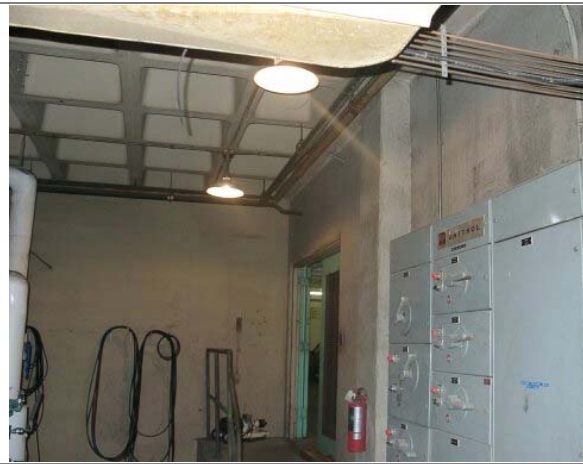
Equipment Room Lights and Power Panels
