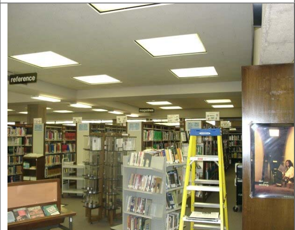
Main Library 4 x 4, 8-lamp Fixtures
