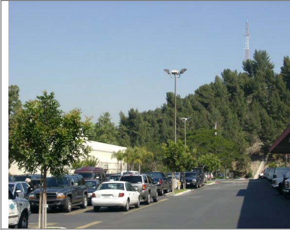
Parking Lot Lights
