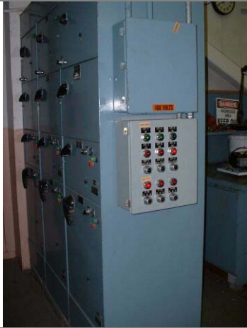
480 V Panel in Boiler Motor Room
