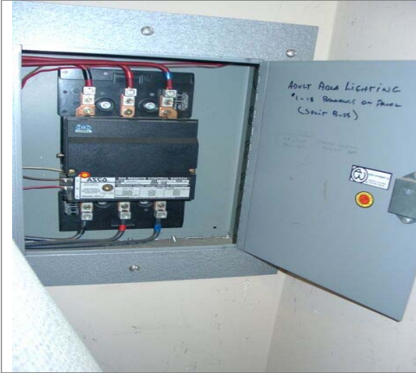
Contactor that feeds top half of panel A
