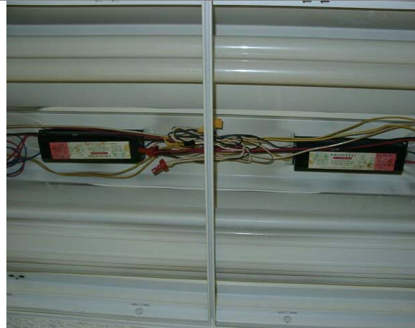
Another Picture of a 4-lamp 4-Foot Fluorescent Fixture With Ballasts
