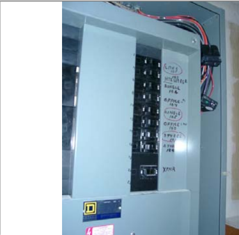
Lighting Panel With Data Logger
