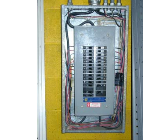
Warehouse Lighting Breaker Panel
