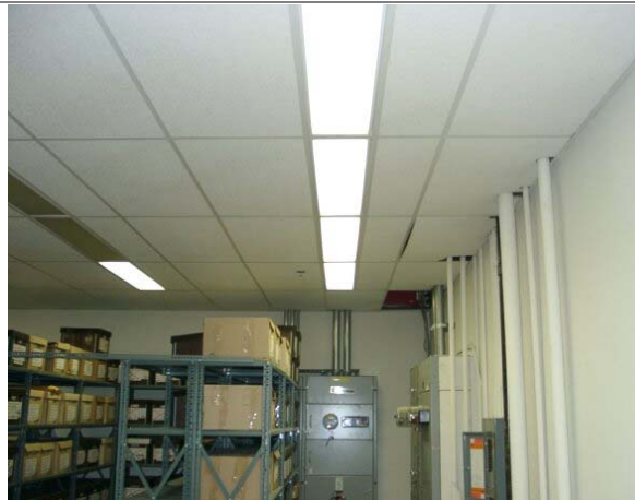
Break Room Lighting Fixtures
