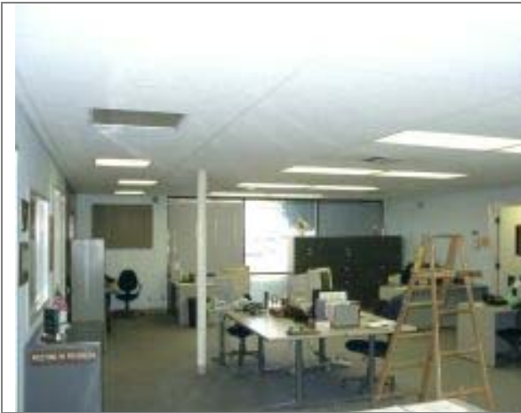
Downstairs Bullpen Lighting Fixtures
