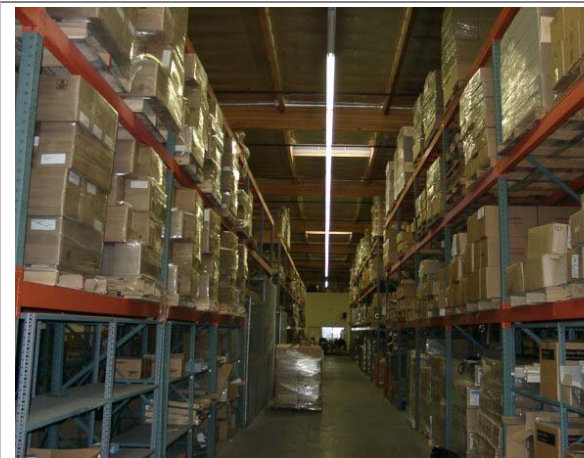
Warehouse Lighting Fixture Row
