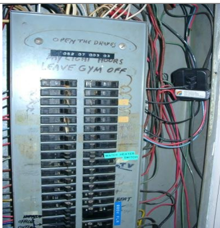
Old Gym Area Breaker Panel With Datalogger
