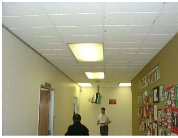
Hallway Light Fixtures
