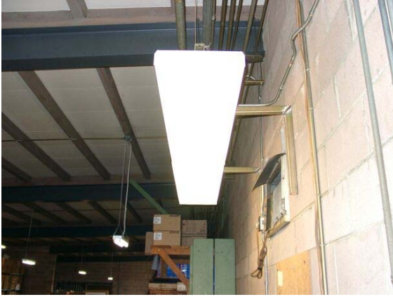
Warehouse 4-lamp Fluorescent Light Fixtures
