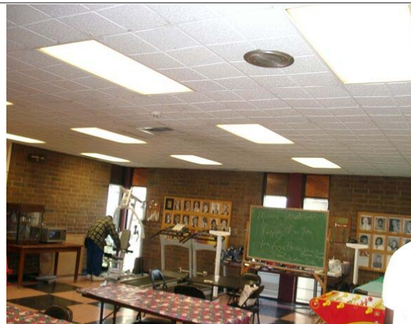
Large Activity Room Light Fixtures
