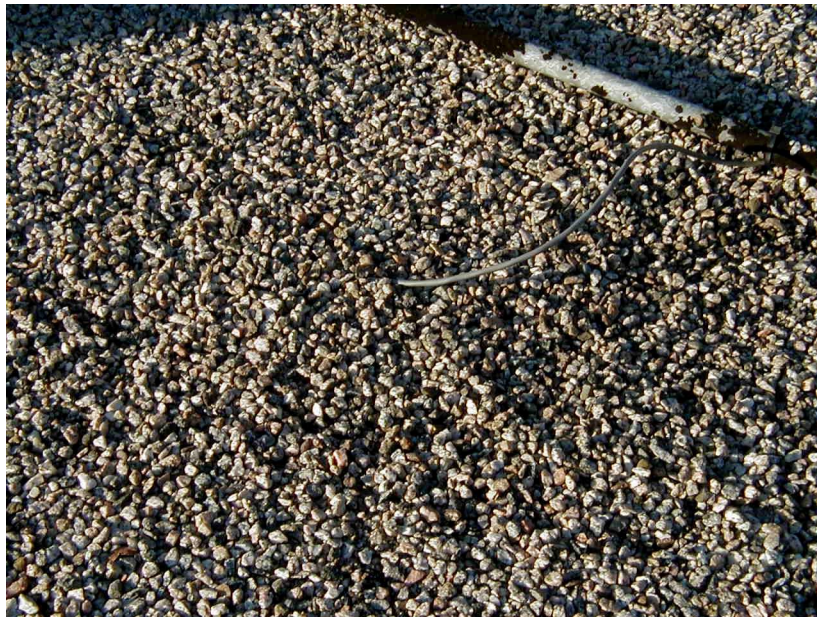
Figure 3. Roof Temperature Sensor
