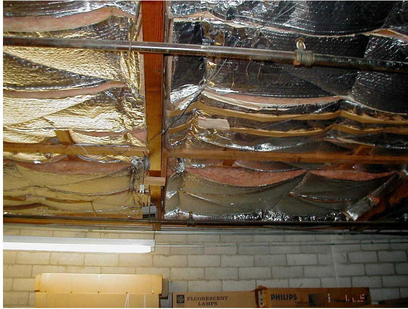
Figure 1. Coated Store Ceiling and Insulation
