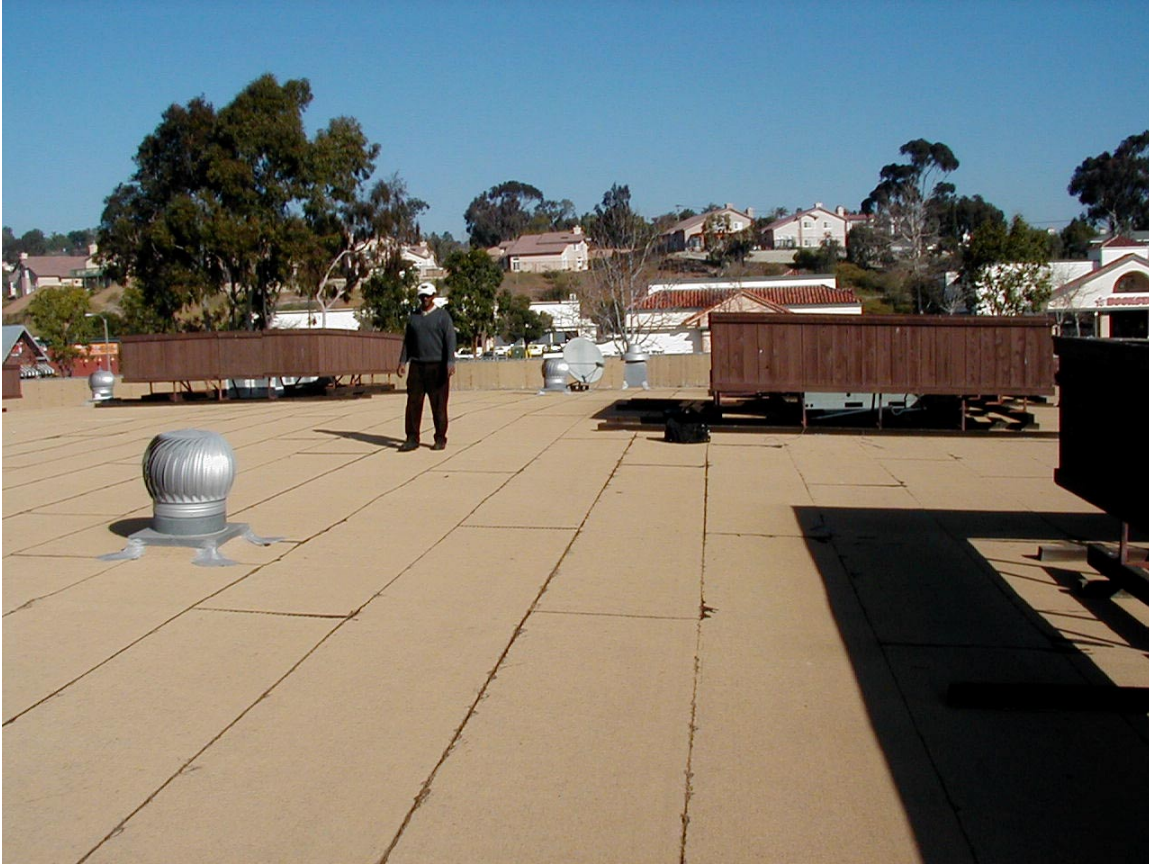
Figure 4. Uncoated Store Roof
