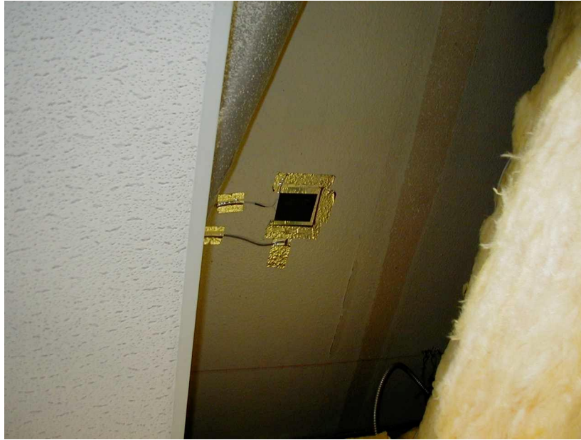
Figure 4. Sheet Rock Instrumentation
