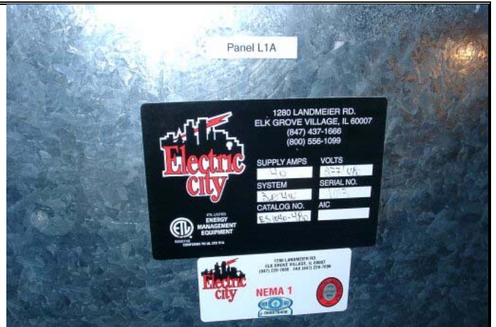
Nameplate for Unit 1013
