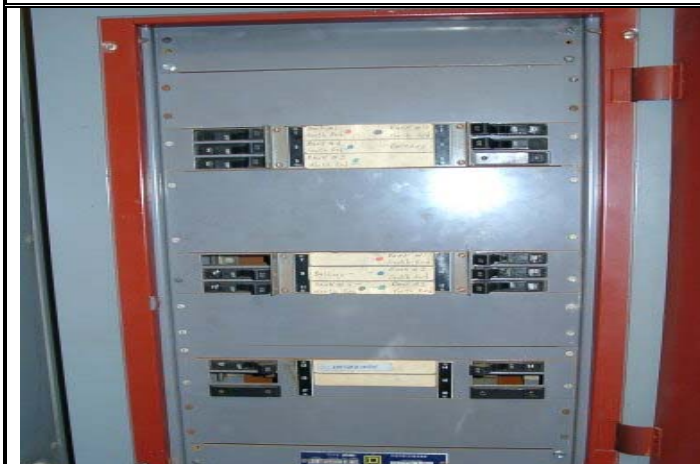
Gym Lights Breaker Panel
