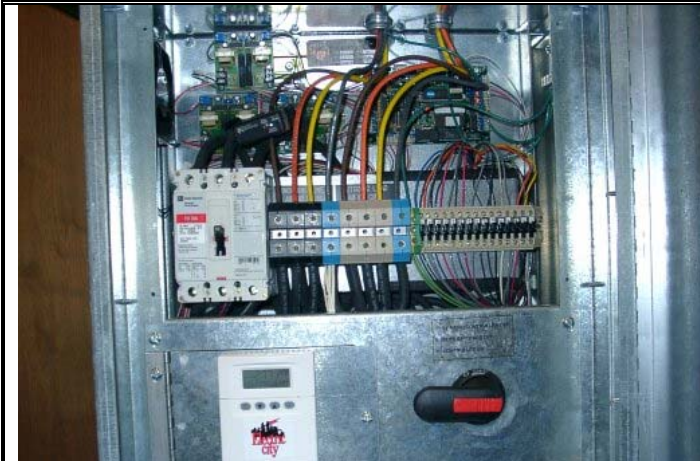
Library 3 rd Floor Unit 964 With Datalogger Installed
