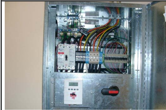
Library Unit 958 With Datalogger Installed
