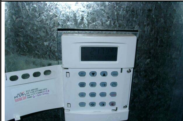
Meter for Unit 983
