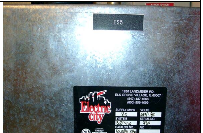
Nameplate for Unit 984
