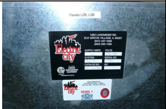
Nameplate for Unit 996
