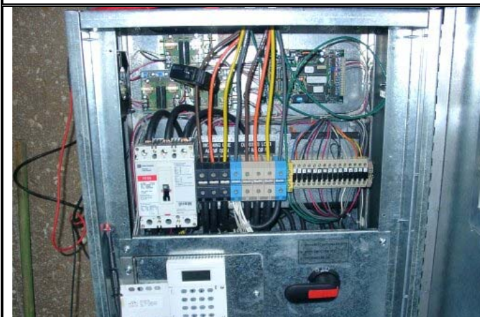
Library 5 th Floor Unit 995 With Datalogger Installed
