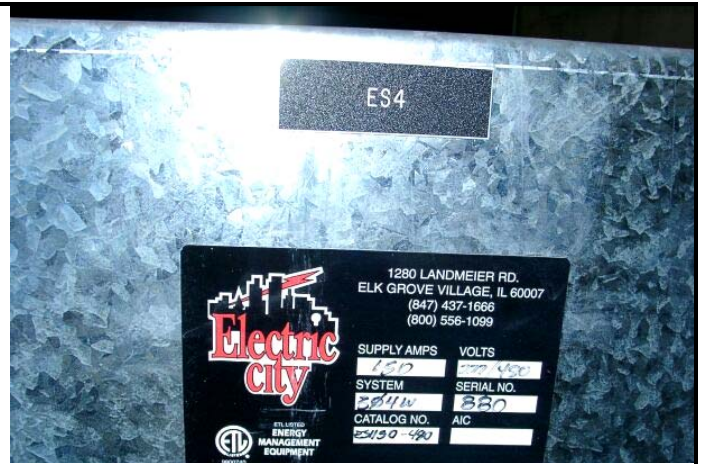
Nameplate for Unit 880
