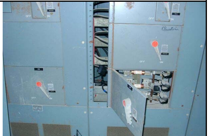
Disconnect for Unit 894
