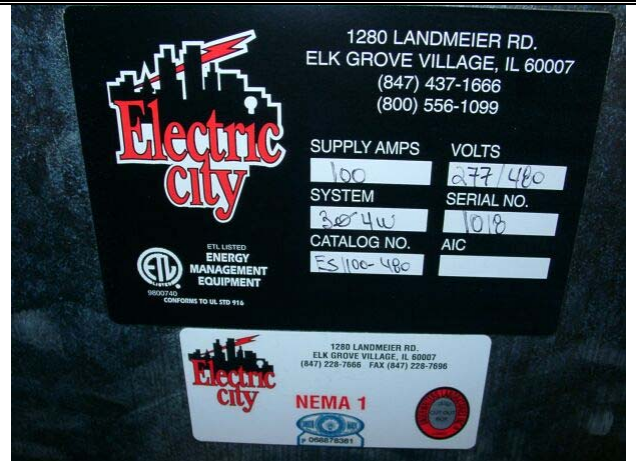
Nameplate for Unit 1018
