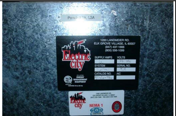
Nameplate for Unit 964
