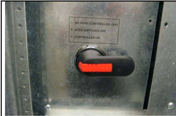
Unit 882 in Bypass
