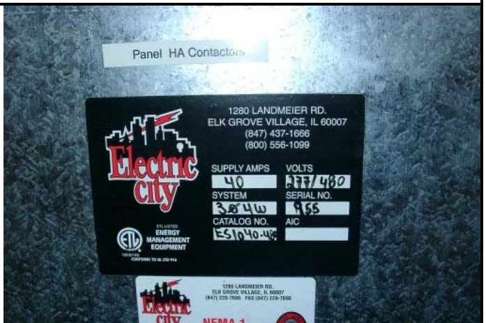
Nameplate for Unit 955
