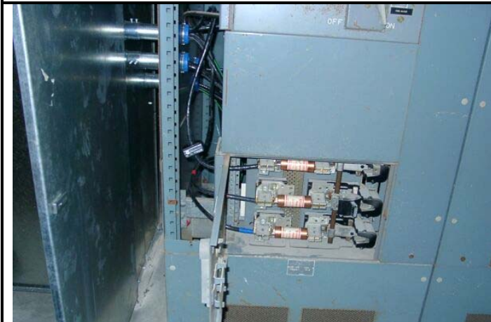
Disconnect for Unit 413
