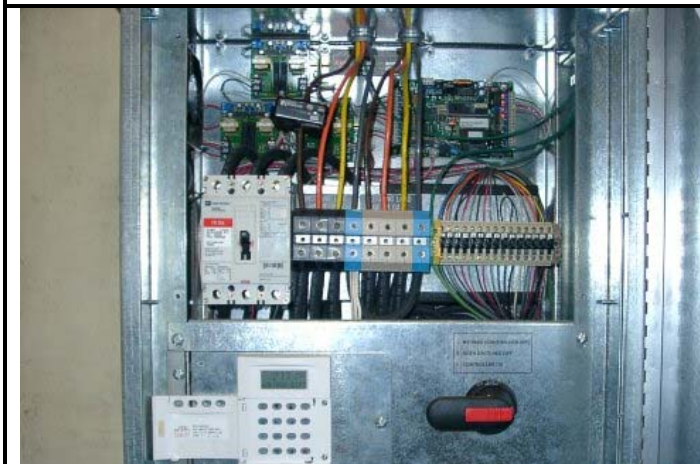
Gym Unit 955 With Datalogger Installed
