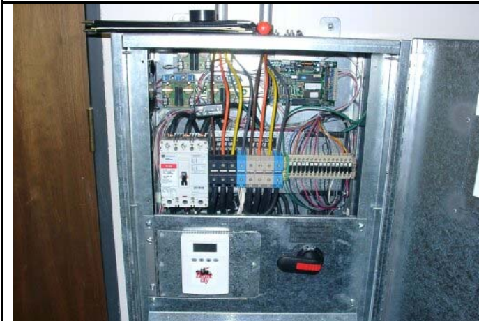
Library 3 rd Floor Unit 996 With Datalogger Installed
