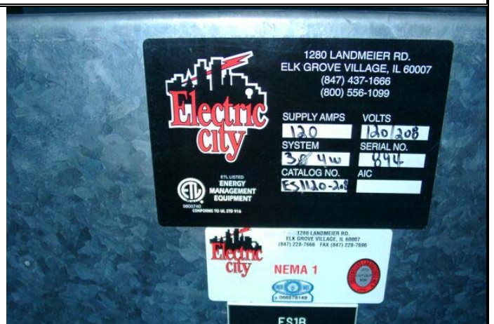
Nameplate for Unit 894
