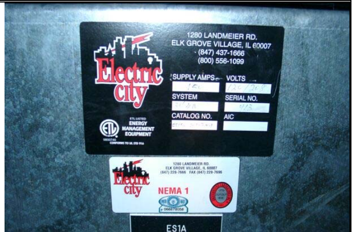
Nameplate for Unit 413
