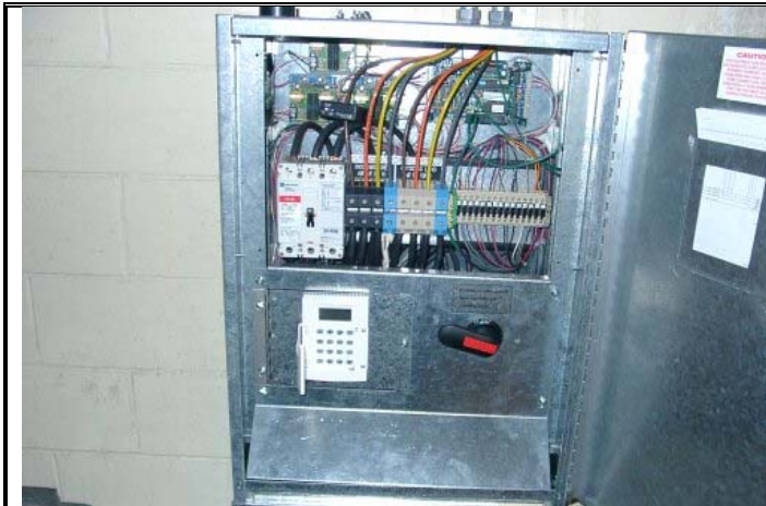
Library Mech. Room Unit 1013 With Datalogger Installed
