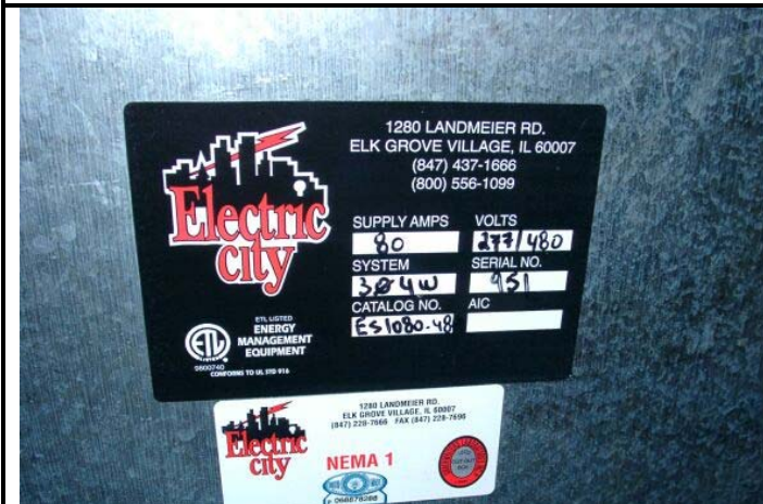
Nameplate for Unit 951
