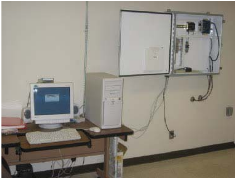
The computer and SCADA control box located within the mechanical room.
