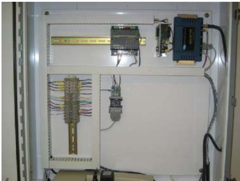
Control panel with three different types of connections: direct connect via Ethernet, RS232 Modem via twisted pair phone line, and radio frequency spread spectrum, 900 MHz.
