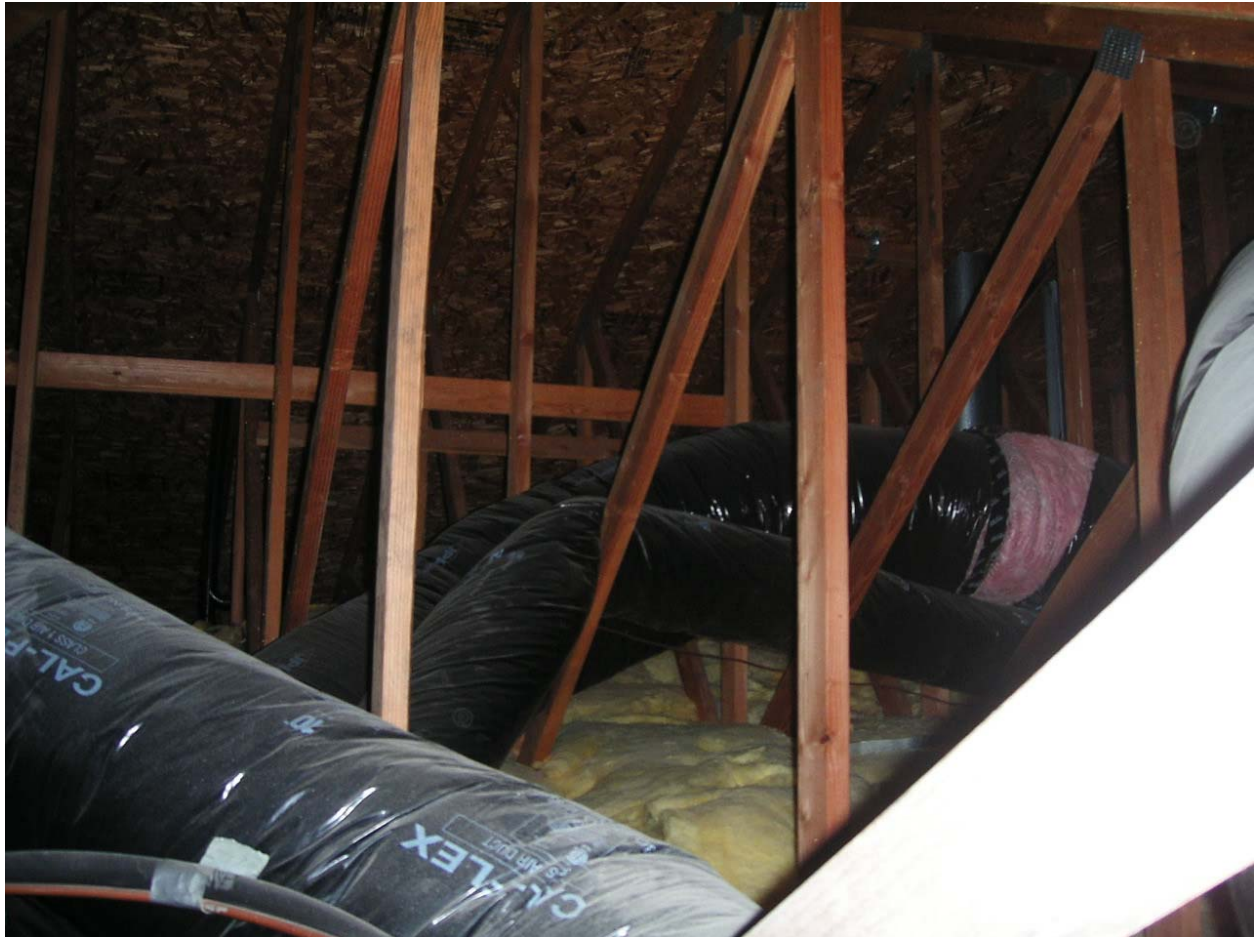
Figure D-4 Kink Consistent with Installation, Retained
