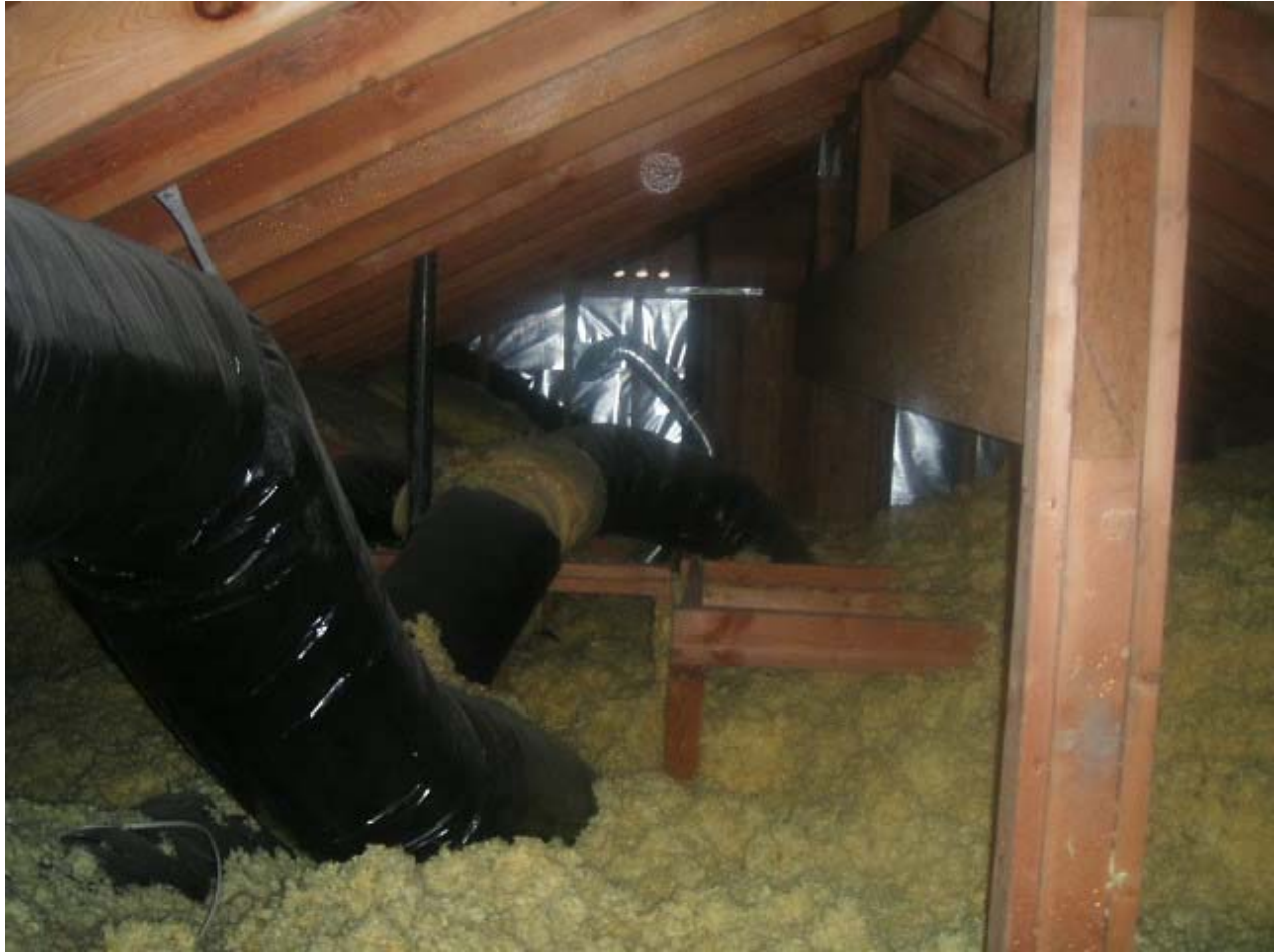
Figure D-2 Nicely Installed Ducts, Retained
