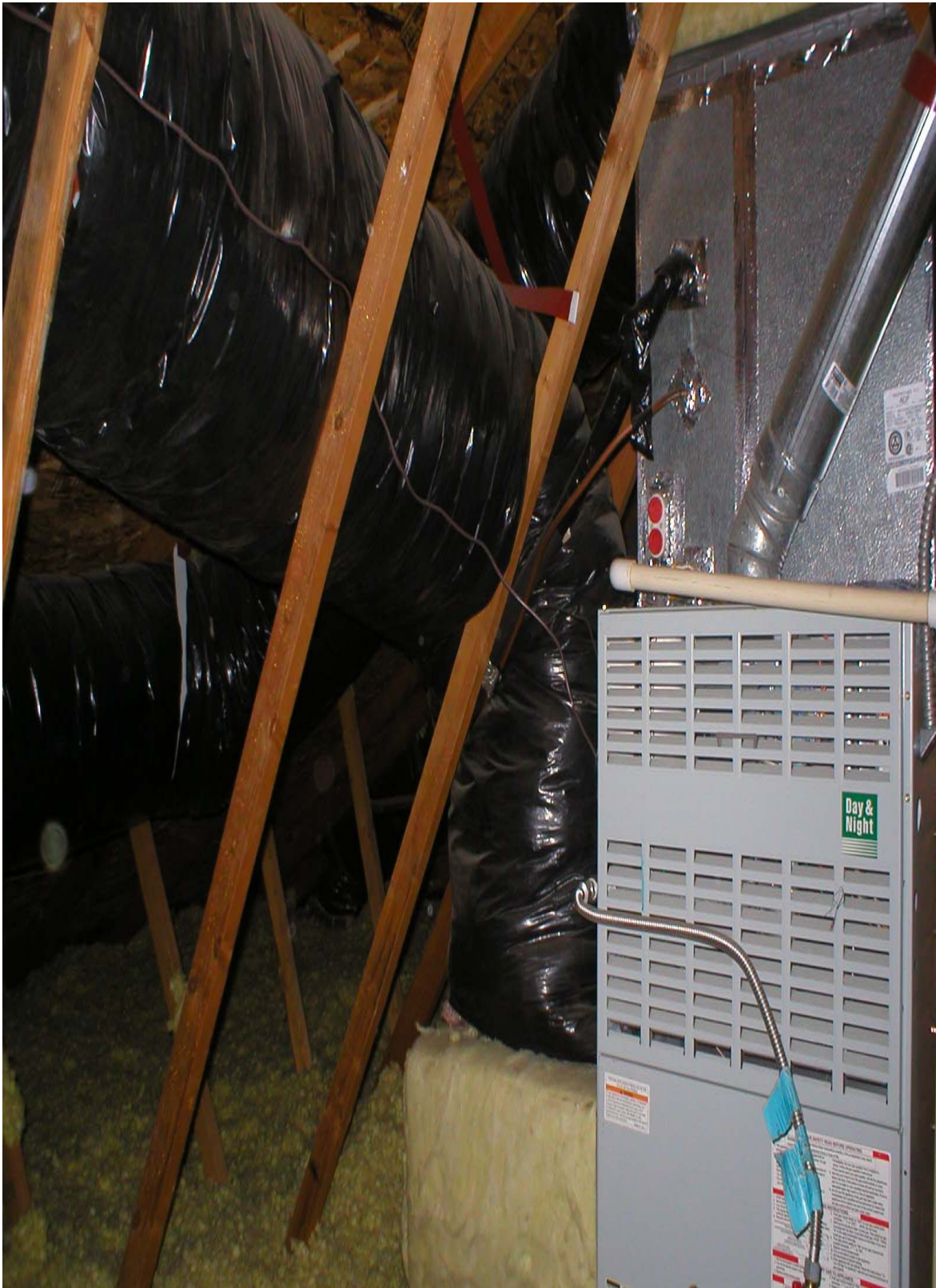
Figure D-3 Nicely Installed Ducts, Retained
