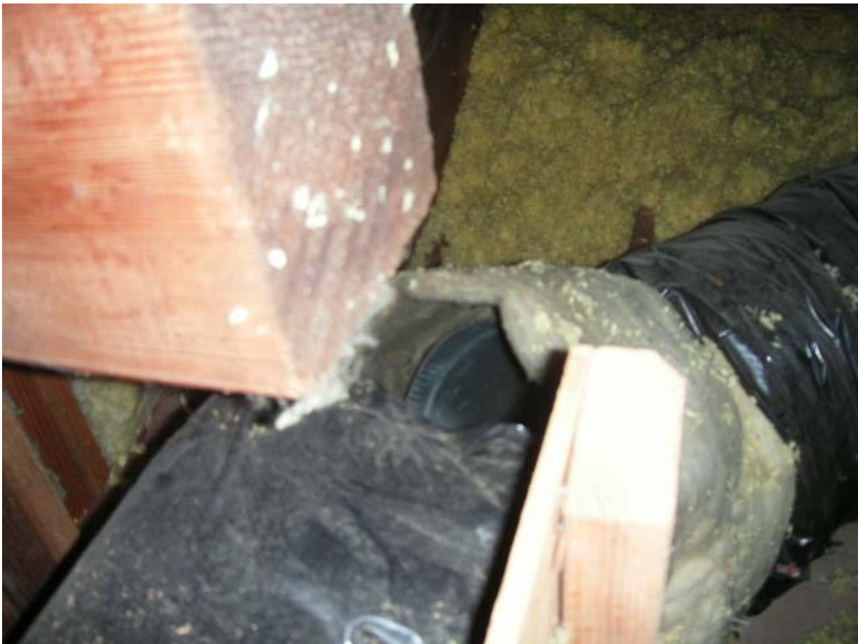
Figure D-1 Disconnected Duct, Non-retention
