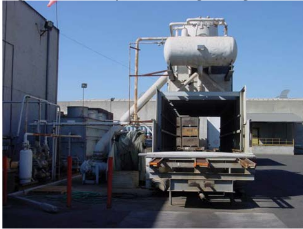
Figure 2.2 Old Hydro-Cooling Refrigeration
