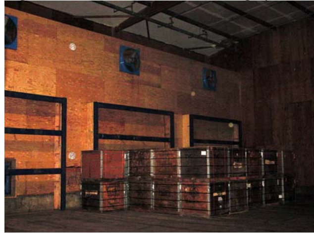
Figure 2.3 New Internal Air-Cooling System
