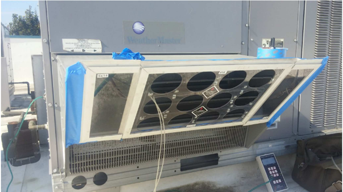
Figure 15. Trueflow outside air measurement set-up
