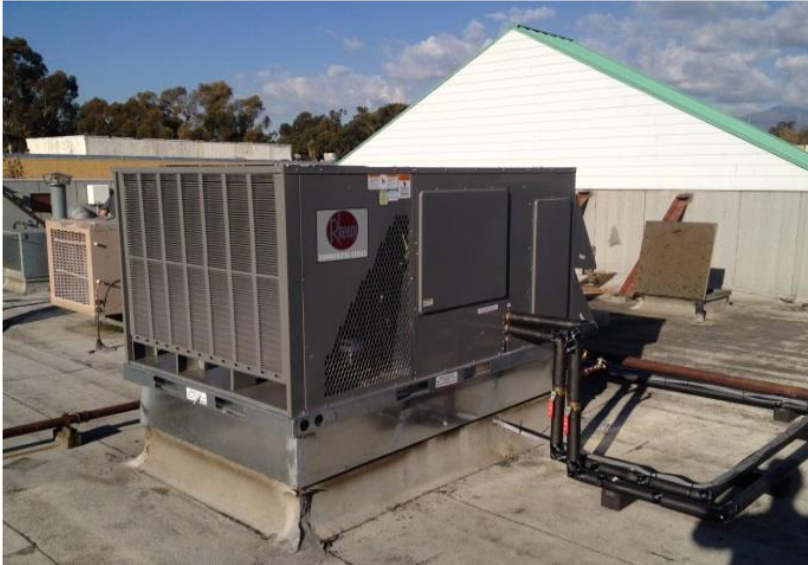
Figure 13 Wasted Heat Recovery Unit 93
