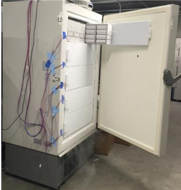
Figure 9. Ultra-Low Temperature Freezer 46
